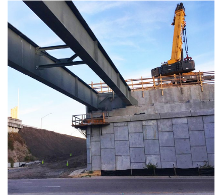
This straight steel I-girder bridge under construction shows key features like the concrete abutment, the I-beams, and a cross frame.
