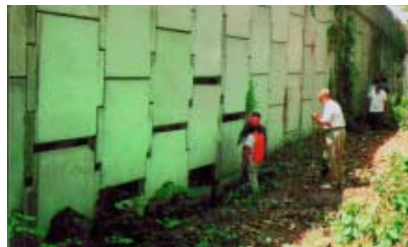
Figure 29, Settlement from Pipe Joint Leakage
