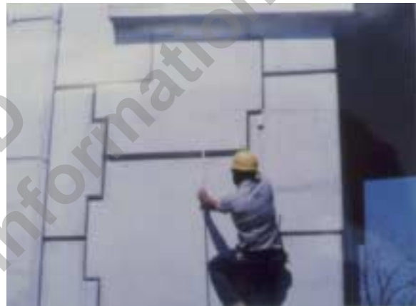
Figure 27, Joints Opening from Settlement
