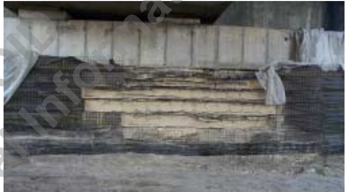
Figure 31, Fire Damaged Reinforcement
