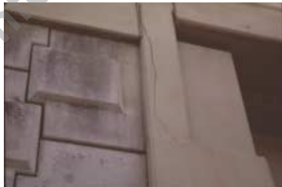
Figure 20, Tension Break in Cheek Wall
