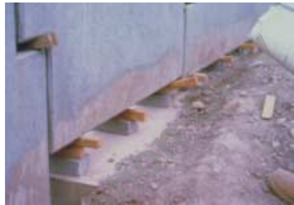
Figure 2, Improper Leveling Pad
