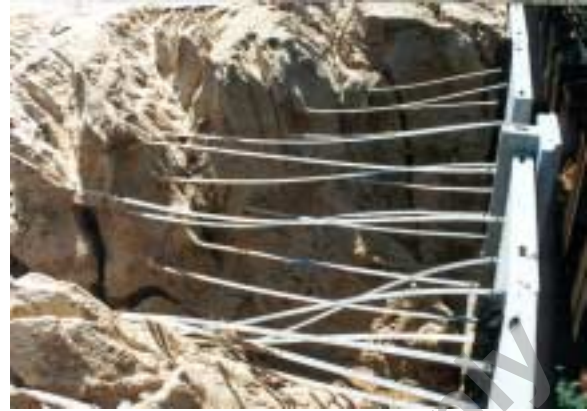
Figure 23, Wash Out From Around Reinforcement
