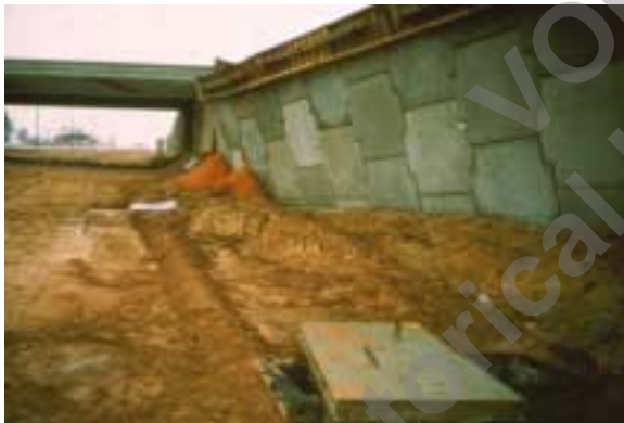
Figure 28, Wall Failure from Exterior Excavation
