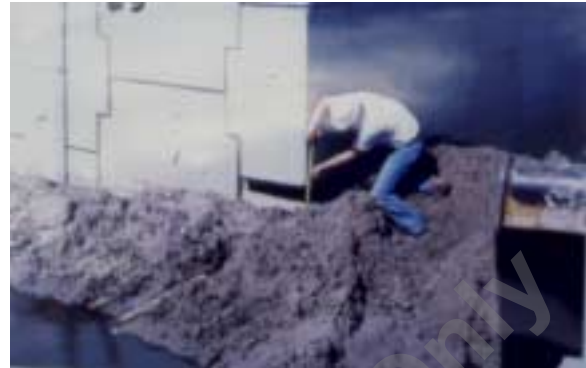
Figure 26, Settlement from Excavation
