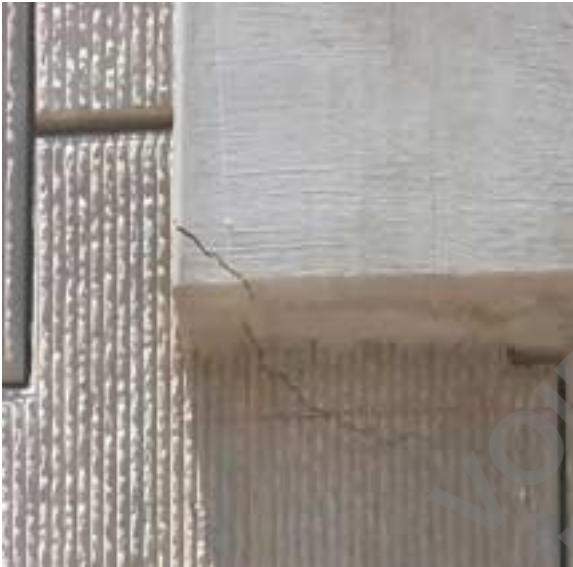
Figure 19, Cracked Panel and Cheek Wall
