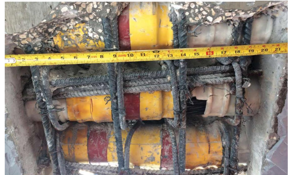
Ultra-high-performance concrete was used for the repair of a midspan spliced U-girder closure pour. Photo: SEMA Construction
