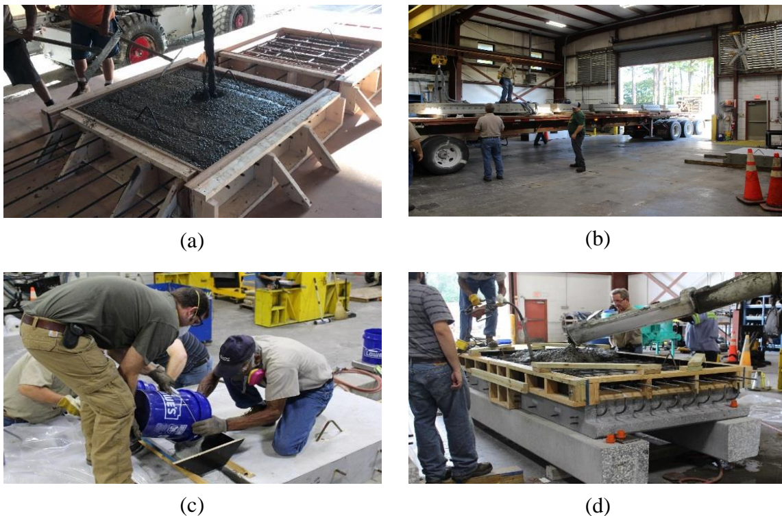
343 344 Fig. 6: Construction of joint specimens: (a) precast specimen concrete pour, (b) delivery of slab- 345 beam specimens to FDOT SRC, (c) casting of field-cast UHPC, and (d) FSB deck casting.
