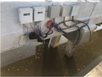
Figure 2.6: Data acquisition modules and wiring
