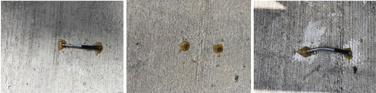
Figure 2.7: Vandalized surface mounted crackmeters
