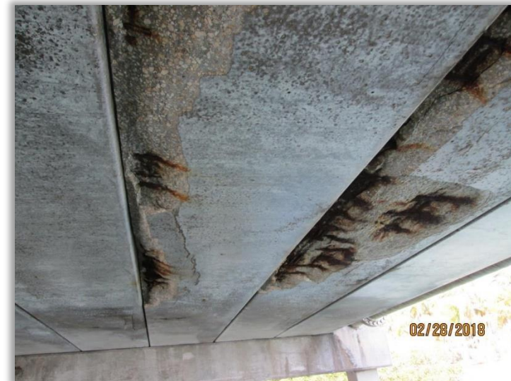
Figure 2: Deterioration on Underside of Slab Units of Spans 3 and 4 (Bridge No 900086)
