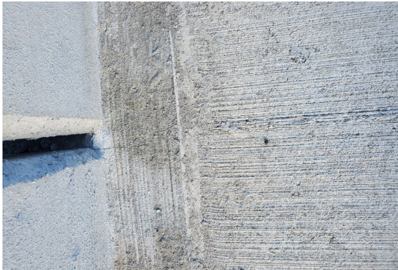
Photo 1: Transverse shrinkage crack in link-slab at centerline Bent 2, showing base of parapet at open joint. Observed in August 2020.
