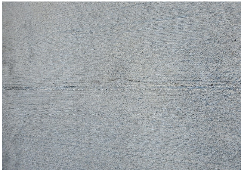
Photo 2: Transverse shrinkage crack in link-slab at centerline Bent 2, showing center of link-slab. Observed in August 2020.
