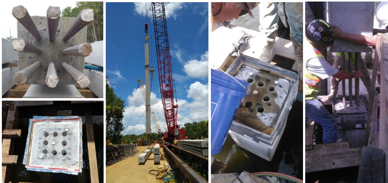
Figure 21-25: Construction of CFCC prestressed splice piles. From left to right the figures display the splice piles, the lifting of the piles, and the epoxy dowelled splice connection.
