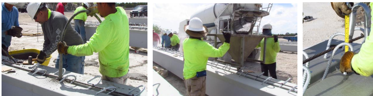
Figures 18-20: HCB compression arch filling process. From left to right the figures display the rubber tipped vibrator, filling of arch using concrete hopper, and tying of shear connectors.
