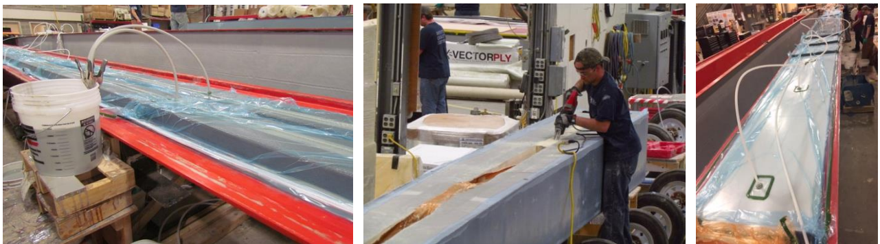
Figure 15-17: HCB resin infusion process. From left to right the figures display the lid infusion setup, the channel being cut into the top of the HCB, and the shell resin infusion setup.
