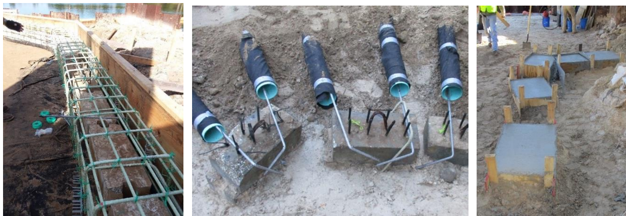
Figures 26-28: CFCC prestressed sheet pile wall tie-back design. From left to right, the figures display the sheet pile wall with GFRP pile cap, installed stainless steel tie-rods in perforated pipe, and formed cast-in-place concrete deadmen anchor blocks.
