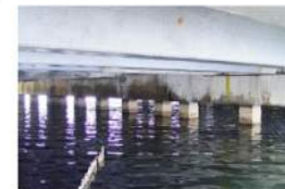
Before its replacement, this bridge developed severe corrosion concerns. The effectiveness of repairs made with FRP was shown in this project.
