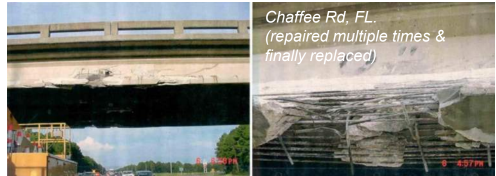
Figure 227—Girder damage from vehicle impact in July of 2001
