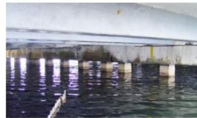
Before its replacement, this bridge developed severe
