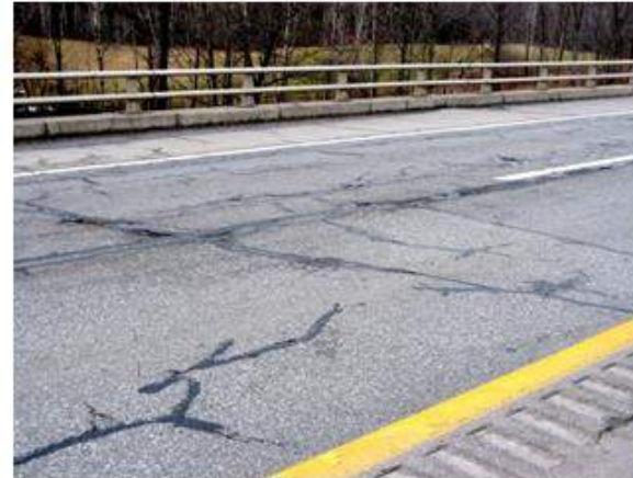
Travel lane exhibit's sev rutting thru iso'l'd potholes.
