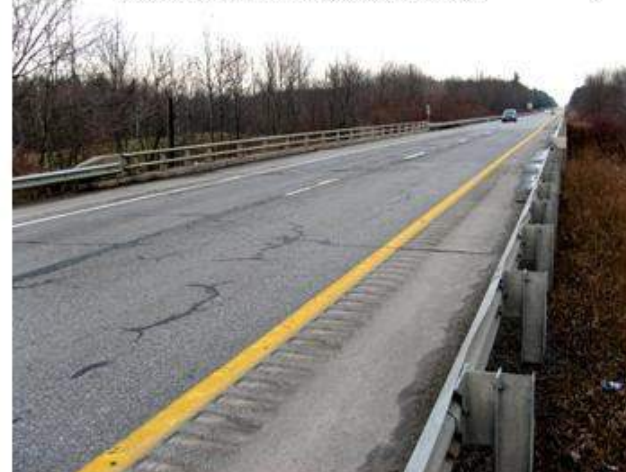
Looking NE'ly against flow of traffic. Apr and wear surf pave deter'd.
