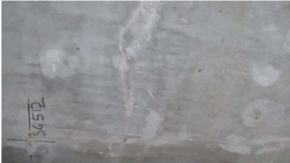
Figure 16: Bottom of slab at construction joint, Span 5, crack near SG512 (at two years)
