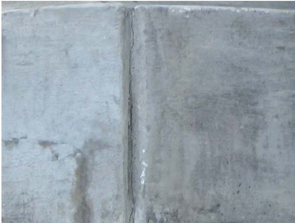
Figure 21: End Bent 6, sheet pile wall cap, vertical crack on north corner of front face
