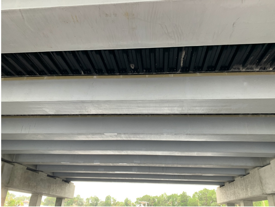
Figure 7: Small gap between HCB lid and vertical face of HCB
