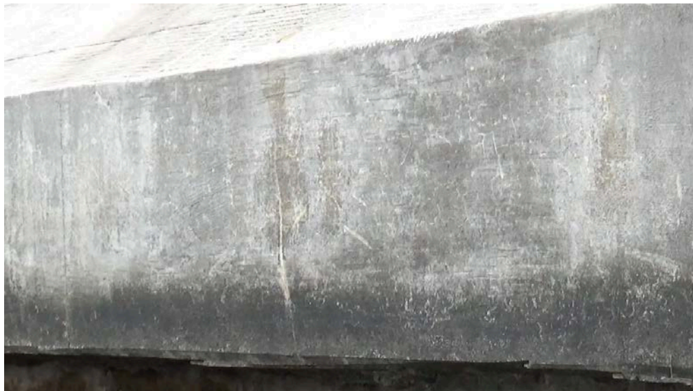
Figure 19: End Bent 6, sheet pile wall cap, vertical crack with efflorescence
