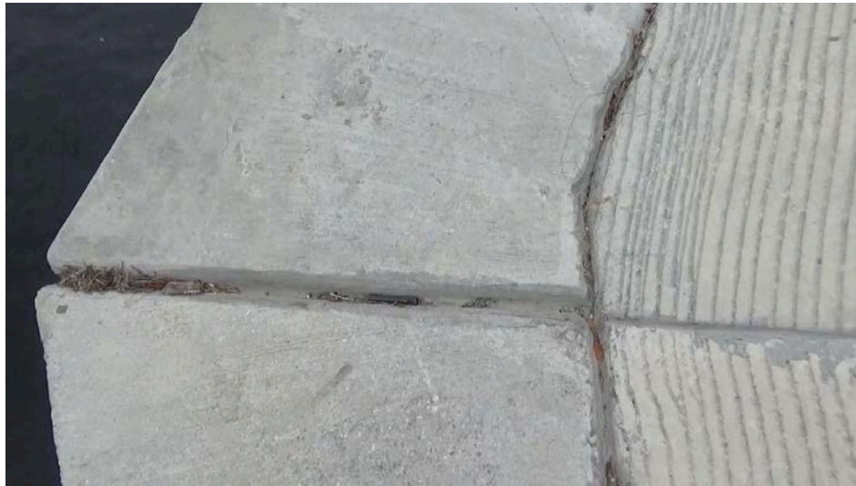
Figure 18: End Bent 6, top of sheet pile wall cap at corner, no cracks (at two years)
