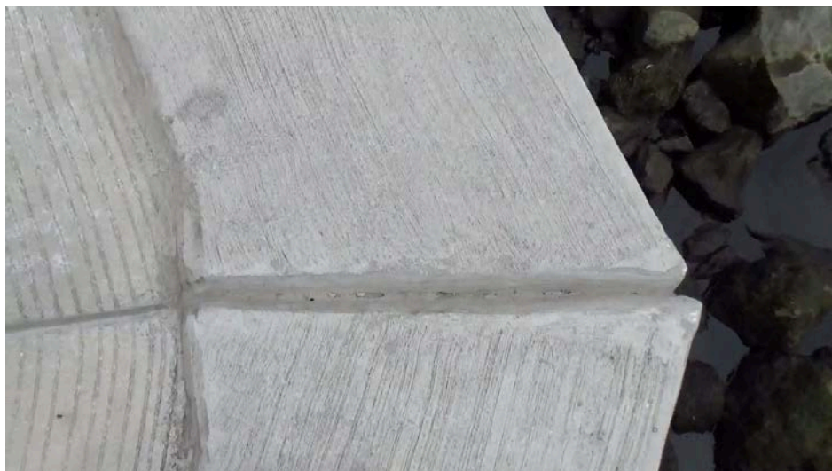
Figure 17: End Bent 1, top of sheet pile wall cap at corner, no cracks (at two years)
