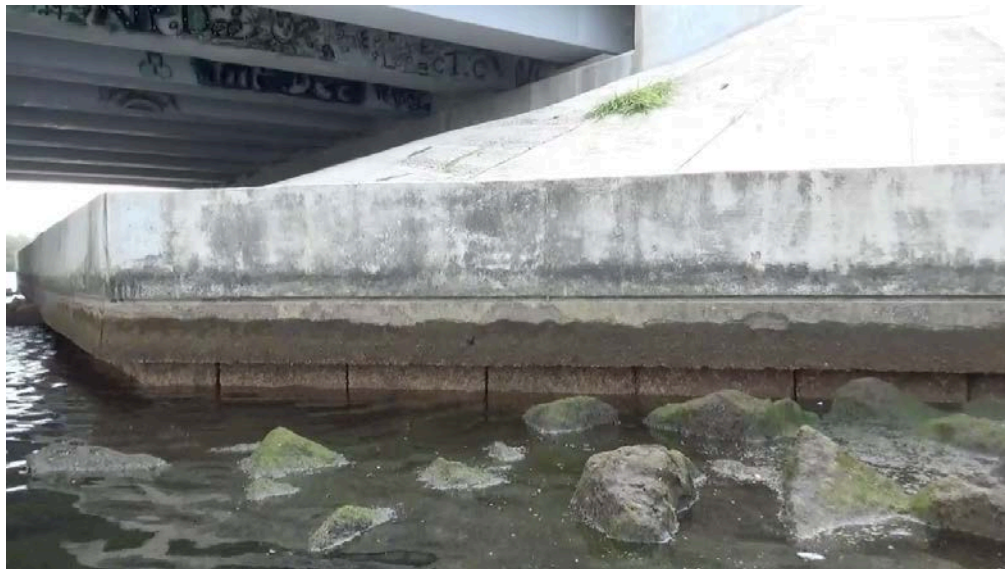
Figure 27: Barnacles on end bent sheet pile wall (at two years)
