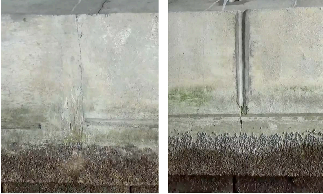
Figure 22: End Bent 6, sheet pile wall cap, vertical cracks at two locations on front face
