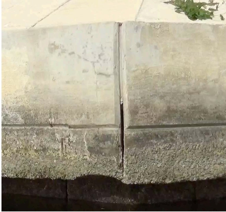
Figure 24: End Bent 6, sheet pile wall cap, joint filler missing on southernmost corner
