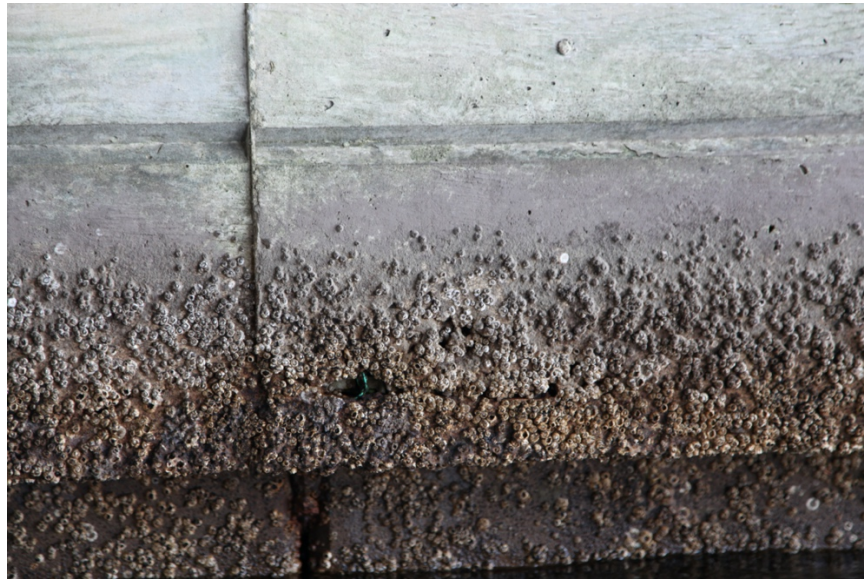
Figure 26: Barnacles on end bent sheet pile wall and cap (at two years)
