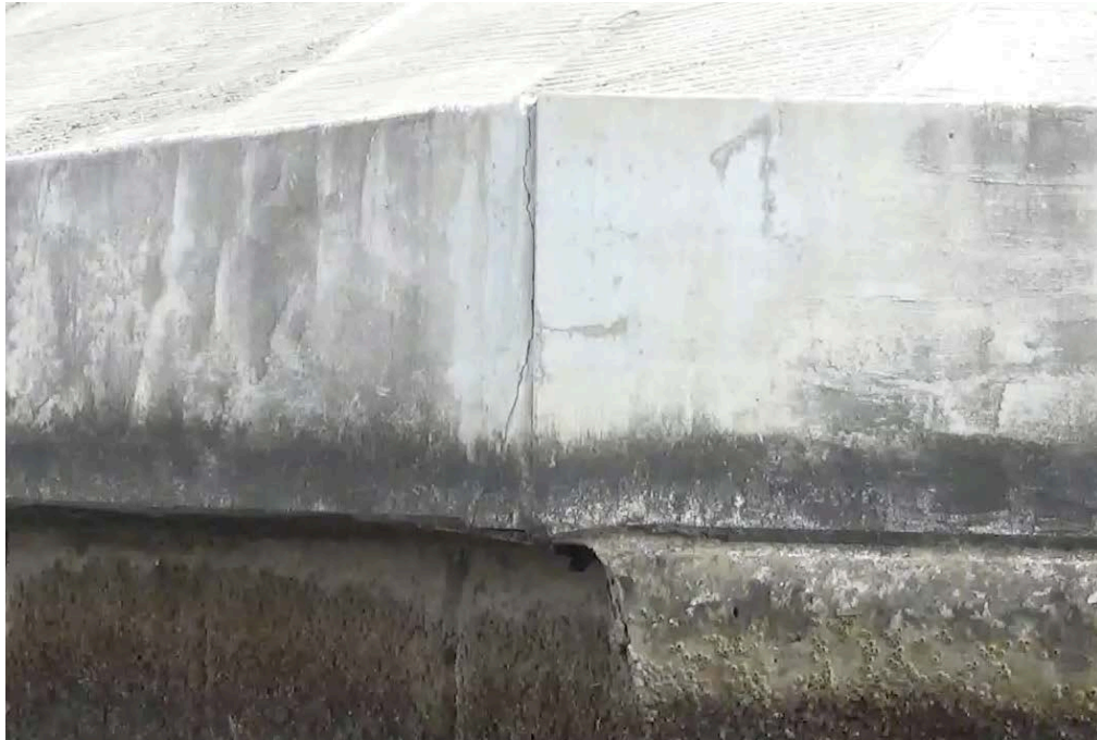
Figure 20: End Bent 6, sheet pile wall cap, vertical crack on northernmost corner
