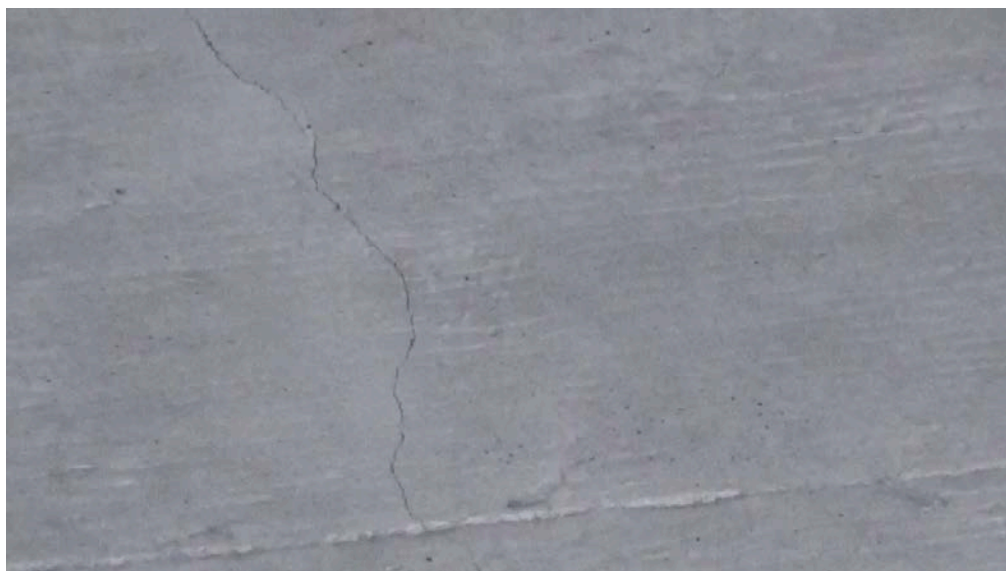
Figure 15: Bottom of slab at construction joint, Span 1, crack near SG112 (at two years)
