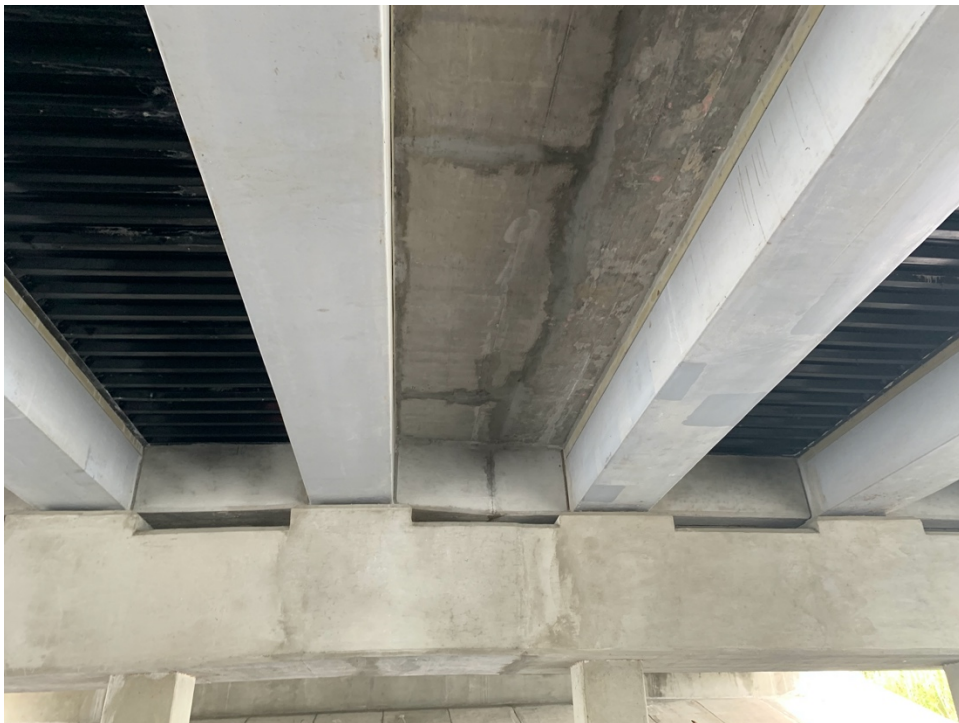
Figure 8: Bottom of slab where connection between construction phases was made, at Bent 2, looking west
