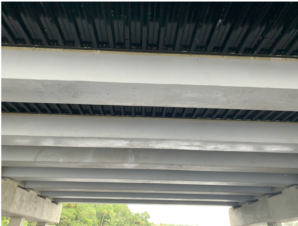
Figure 6: Span 4, gel coat patches on HCB beams
