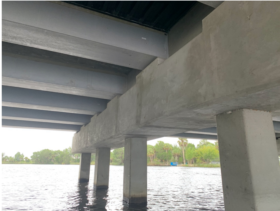
Figure 4: Bent 2, looking northeast, minor staining on bent cap from water drainage
