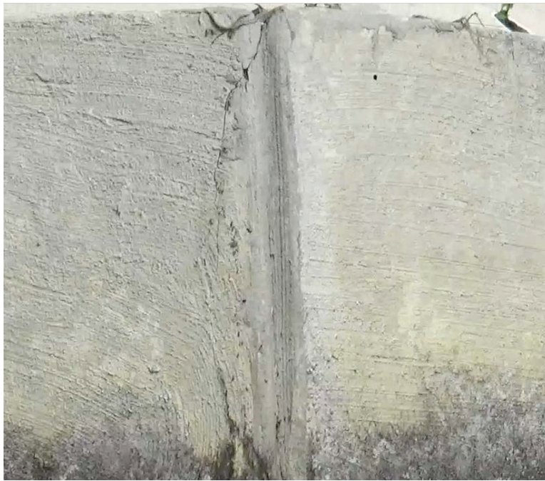
Figure 23: End Bent 6, sheet pile wall cap, vertical crack on south corner of front face
