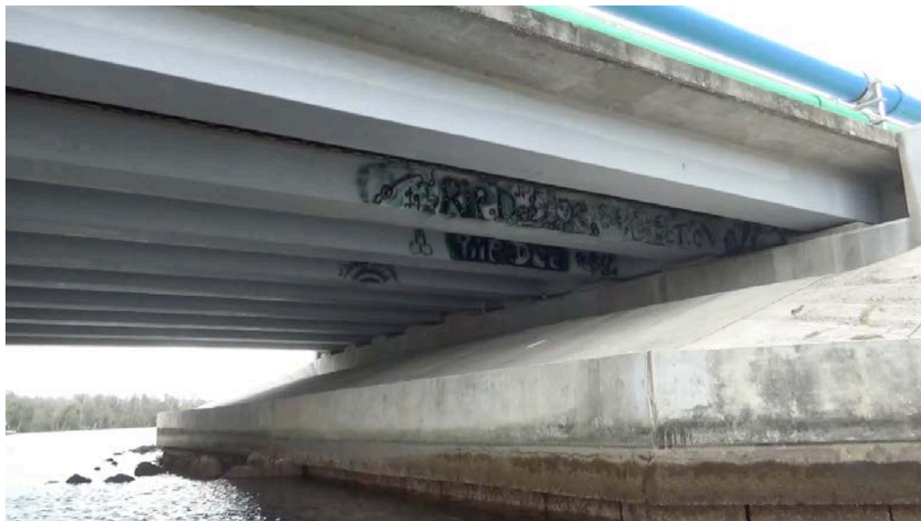
Figure 25: Graffiti on beams above Bent 1, looking southwest (at two years)
