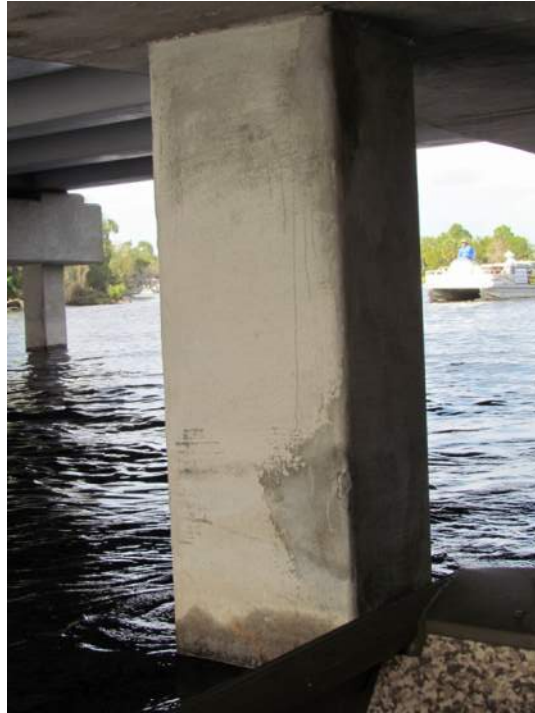
Figure 36: Bent 5 at 3 months, looking northwest; pile discoloration
