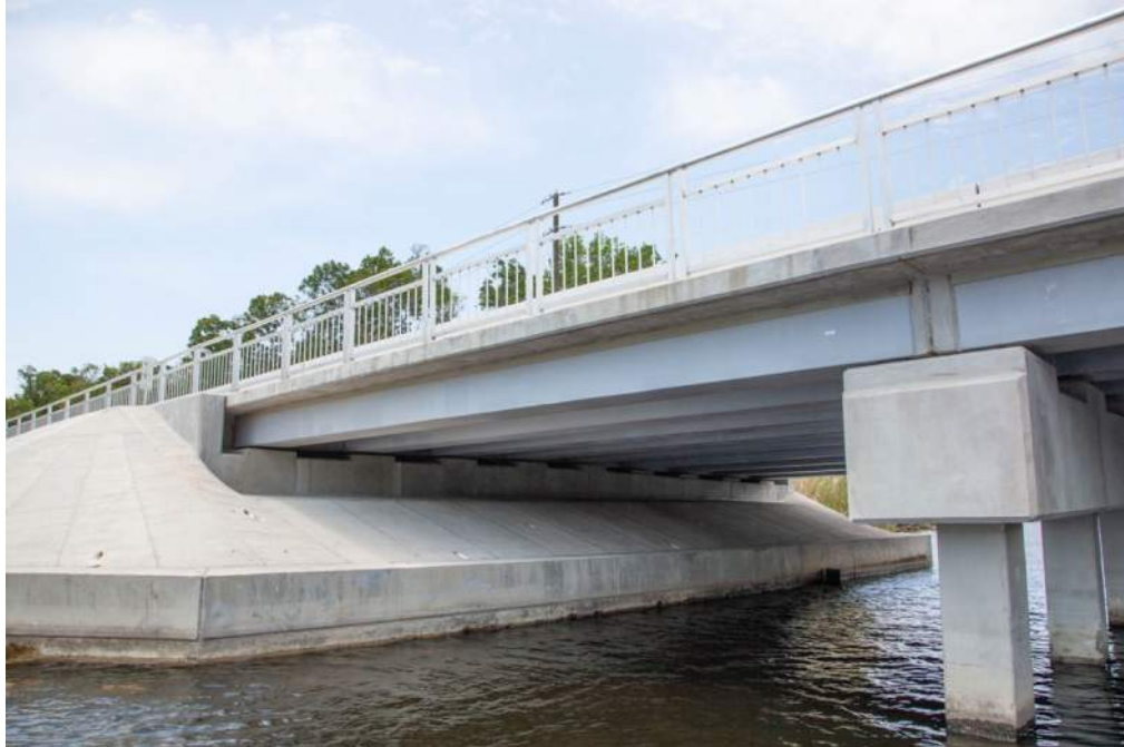
Figure 17: Span 1, looking northwest at End Bent 1 and Bent 2, view from south side
