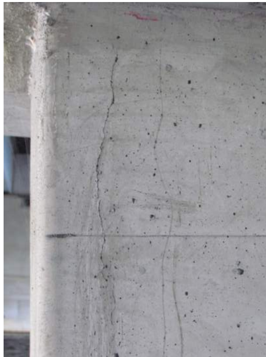
Figure 2: Crack on CFCC pile
