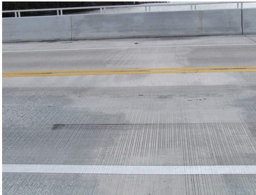
Figure 9: Rough area on roadway
