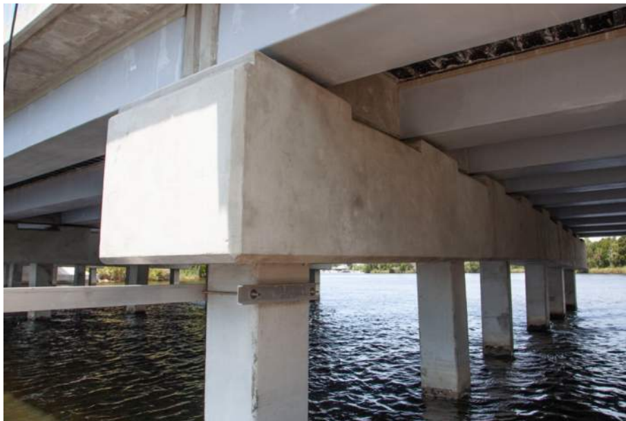
Figure 37: Bent 5 at 6 months, view from south side, looking northwest; pile discoloration (third pile from foreground)
