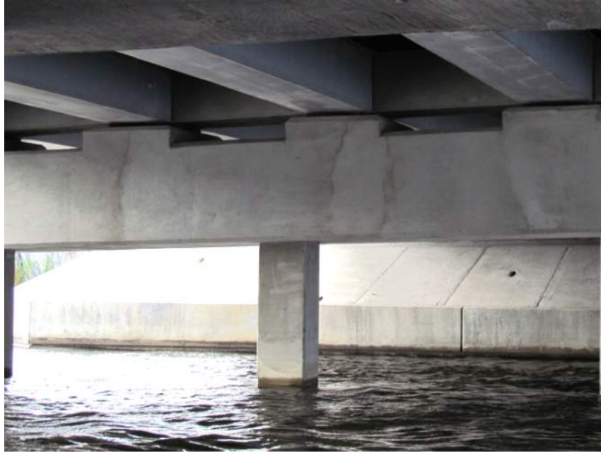
Figure 3: Staining from water drainage
