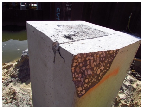
Figure 17: Cracking between CFCC (Bent 1 Pile 2)
