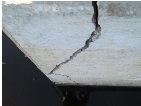
Figure 85: Crack on face of seawall 2B-3B
