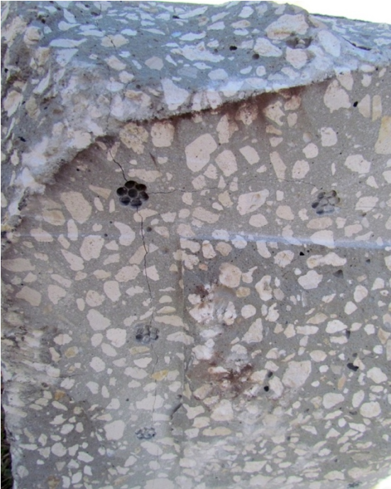
Figure 9: Pile R1 cutoff cracking between strands
