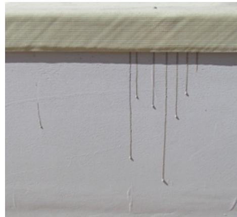
Figure 153: Dripping sealant on HRB-02
