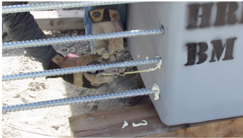
Figure 129: Foaming of diaphragm reinforcement
