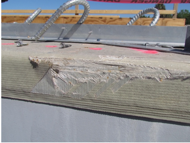
Figure 158: Damaged HCB lid
