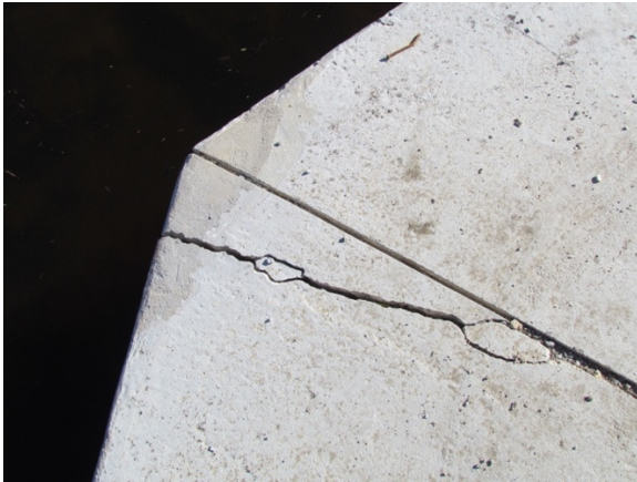
Figure 84: Crack on top of seawall 2B-3B
