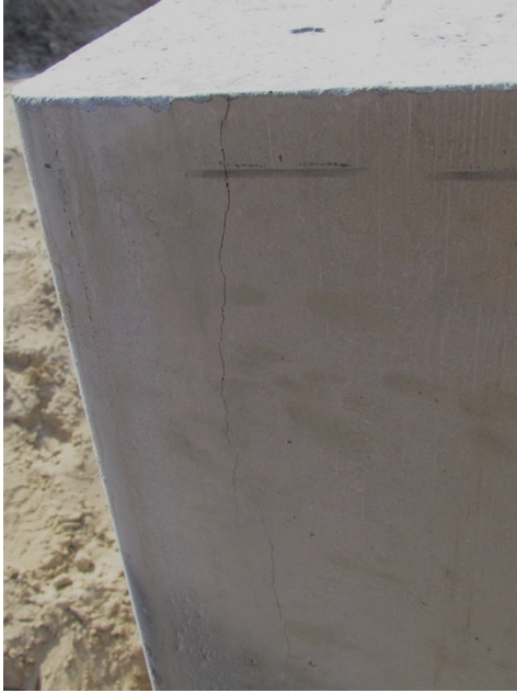
Figure 12: Cracking of Pile 1 at Bent 6
