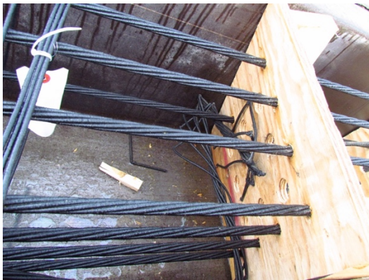
Figure 32: Broken CFCC strand
