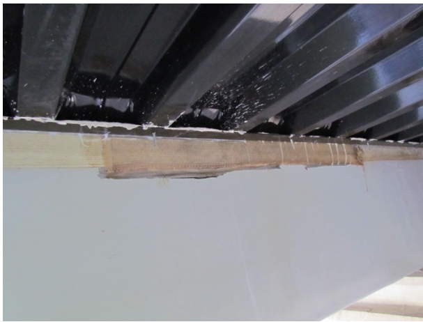
Figure 160: HC Beam patch
