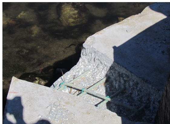
Figure 87: Crack on face of seawall 2B-3B
