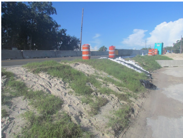
Figure 200: Erosion control on east side of bridge
