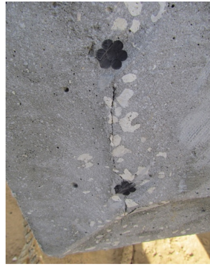
Figure 58: Cracks on piles for Bent 6
