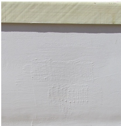
Figure 152: Abrasive patch on HRB-02
