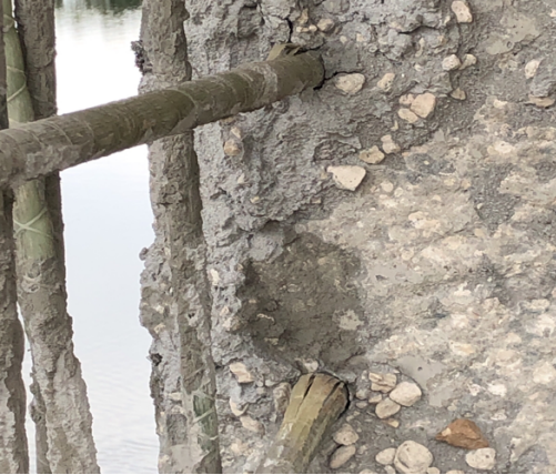
Figure 108: Damaged 8A1 GFRP bar
