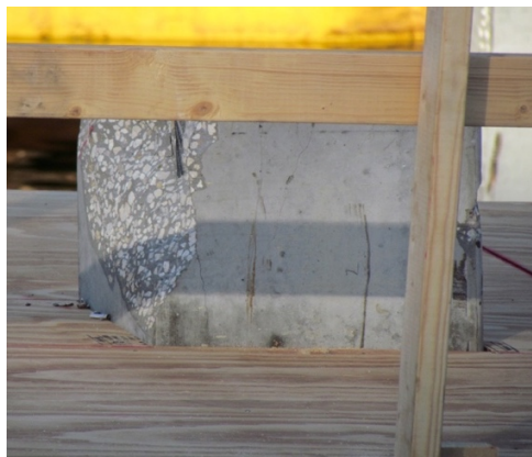
Figure 11: Spalling of Pile 2 Bent 5
