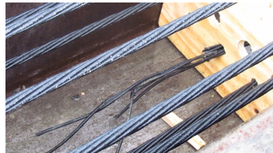
Figure 33: Broken CFCC strand
