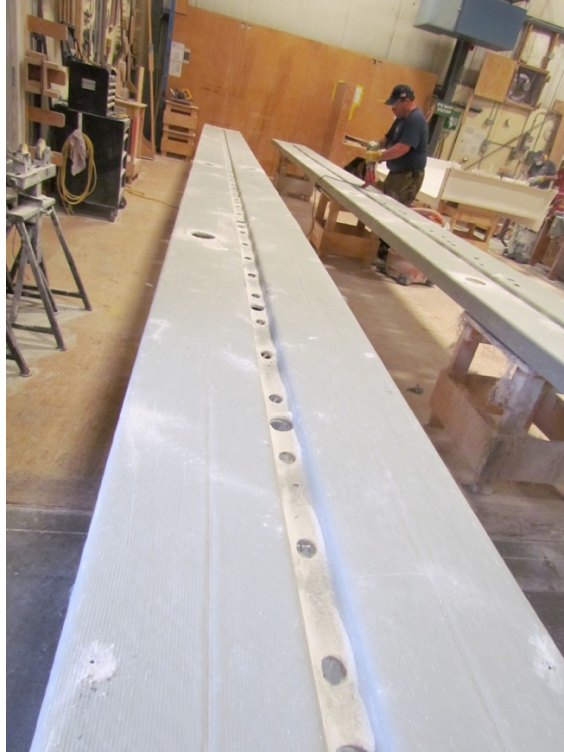
Figure 126: Holes drilled into FRP lid
