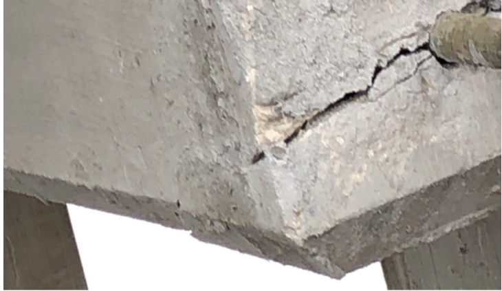
Figure 109: Crack along bottom row of GFRP bars
