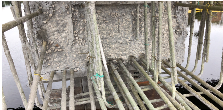
Figure 110: Damaged Pier Cap 4
