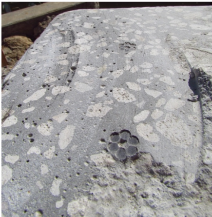
Figure 16: Spalling of Bent 1 Pile 2
