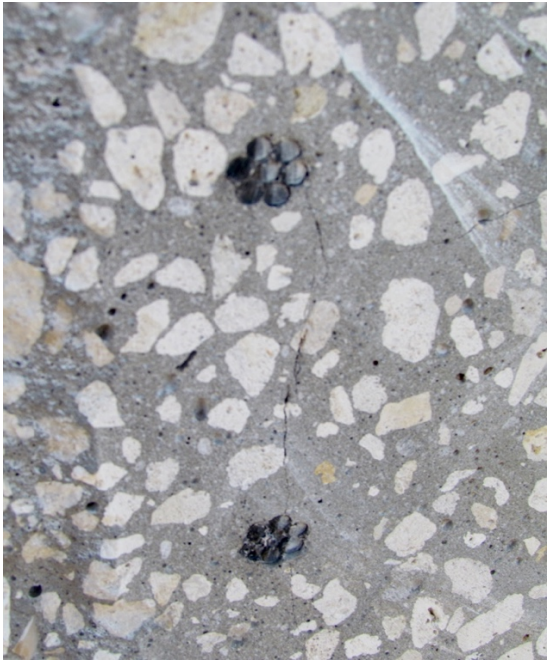
Figure 10: Pile R2 cutoff cracking between strands
