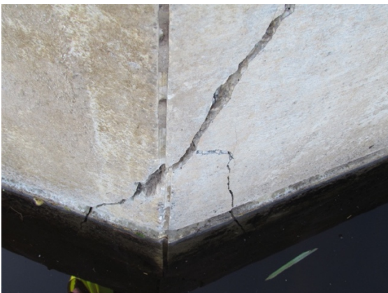
Figure 86: Cut out crack on walls 2A-3A
