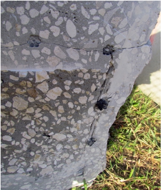
Figure 7: Cracking on Pile R13 cutoff
