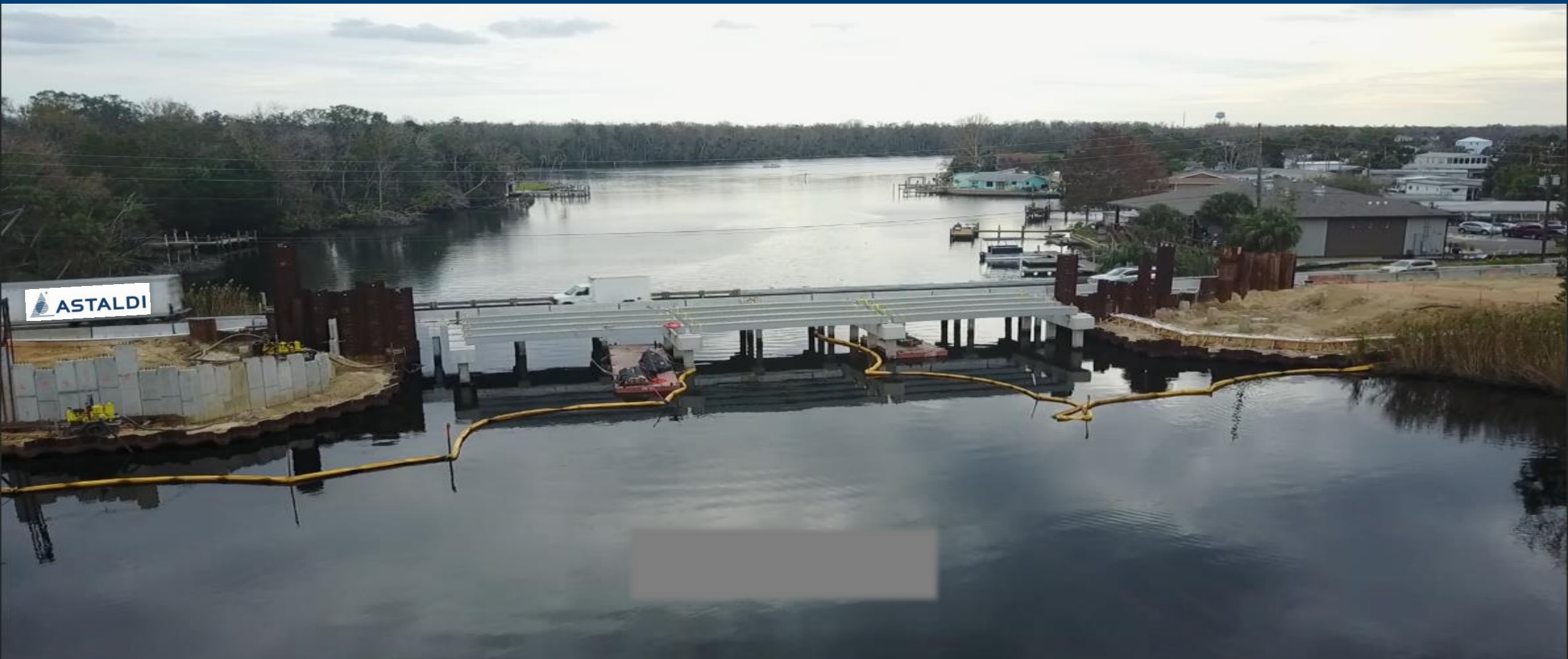
Photo Courtesy of Astaldi Construction Corp. – Halls River Bridge under construction (FDOT FRP-RC/PC & HCB Demonstration project), February 2018.
