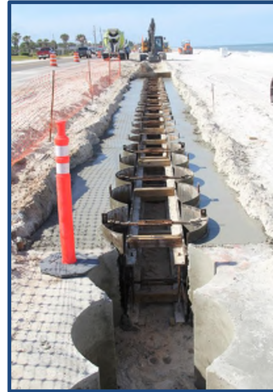
Concrete pouring, i.e. flowable-fill was placed to complete the Secant-Pile layout locations
