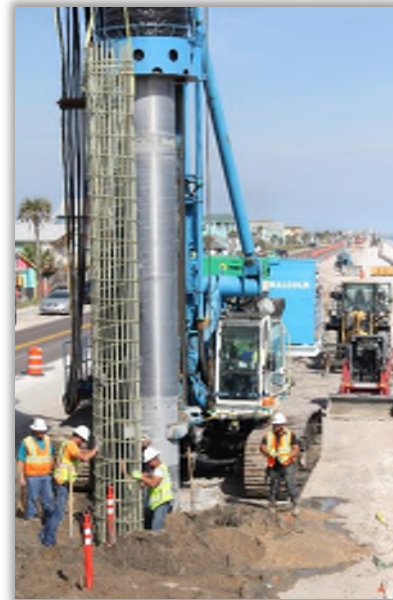
It should be noted that all pile centers have an accuracy of within 1-1/2 in (38 mm) in plan
