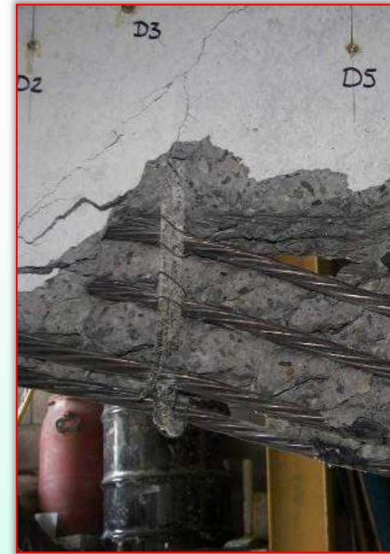
Shear Failure of SC-9.5-2 (CFRP @ d/2 )
