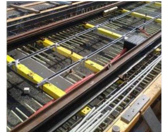
Detector loop at Goldcoast Light Rail project
