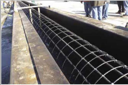
Prestressing bed with carbon-fiber-composite cable strands/spirals for piles for the Nimmo Parkway bridge in Virginia.
