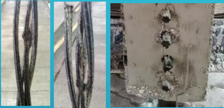
(a) & (b) CFRP strand failed during tensioning; (c) cracking following strands release.
