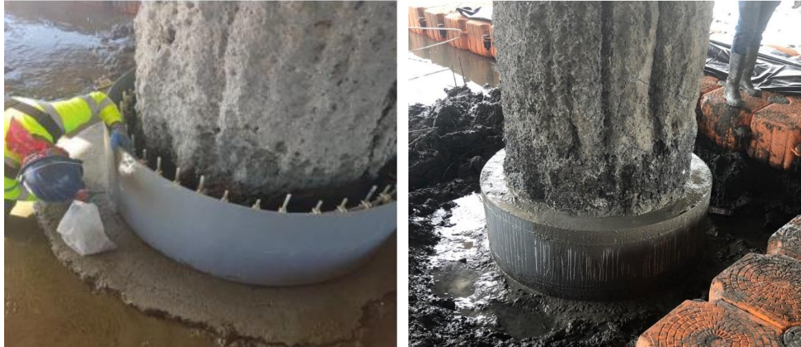
FIGURE 4: Left: reinforcement and jacket before concrete placement of column base, Right: finished column base
