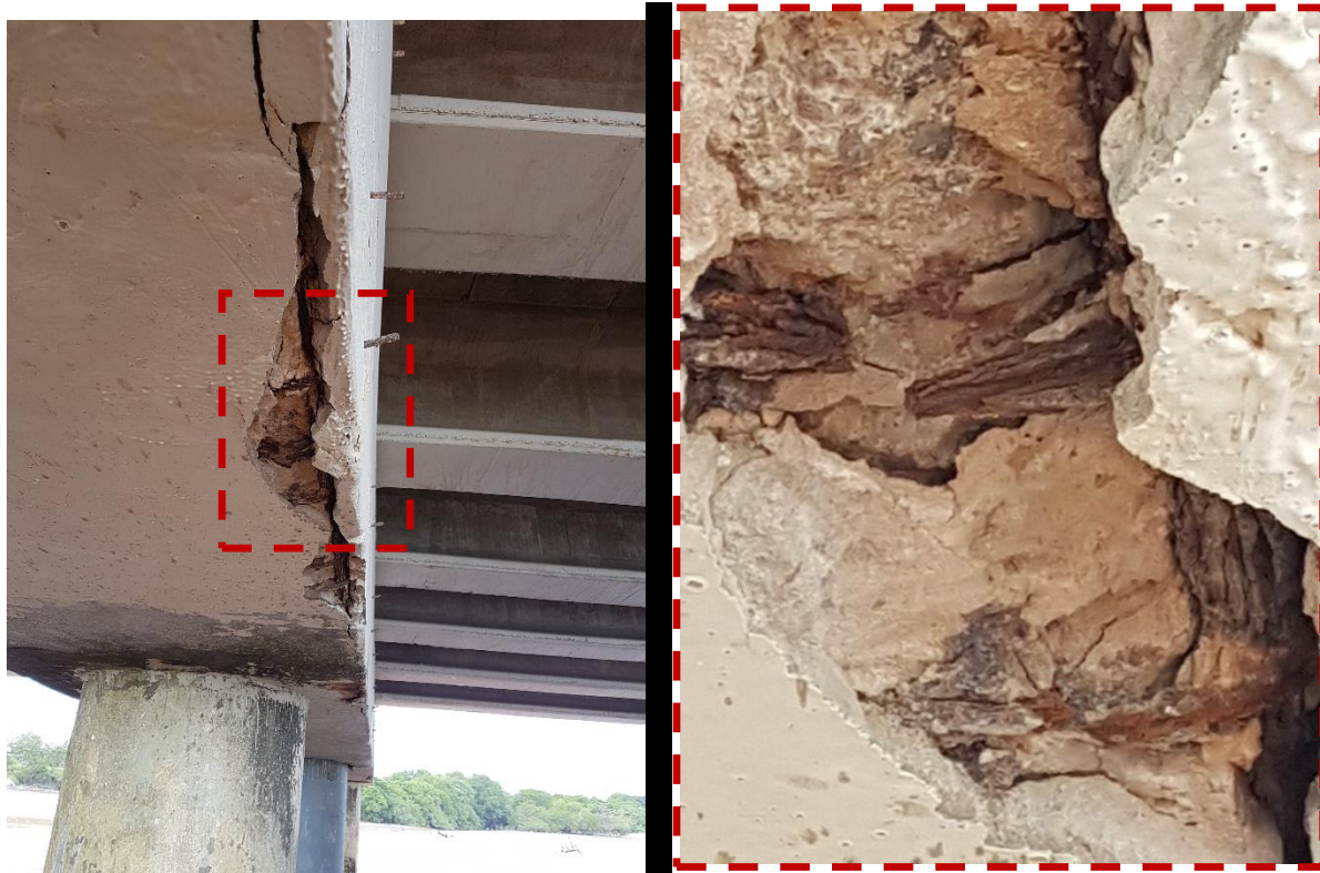
FIGURE 7: Left: damage at underside of bent caps, Right: close-up of broken corner of stirrup
