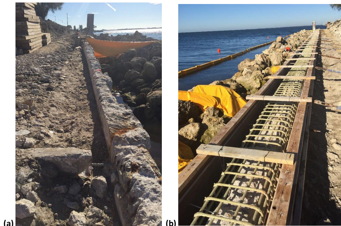
FIGURE 3. (a) Demolition of existing caps showing deep corrosion damage; (b) GFRP rebar replacement caps ready for concrete casting.
