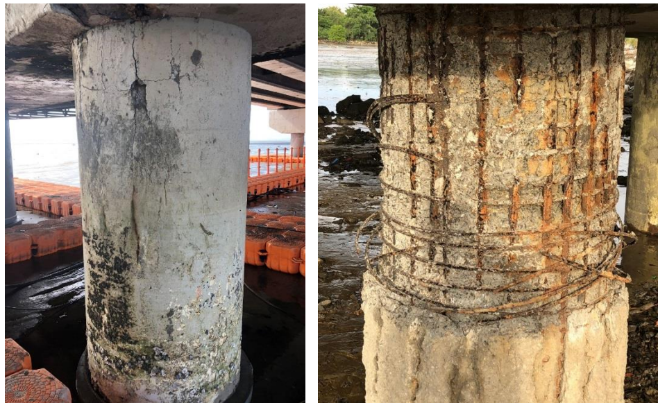
FIGURE 3: Left: Initial condition of columns, Right: Column after cover removal through hydrodemolition
