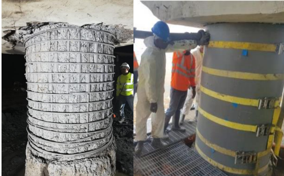
FIGURE 6: Left: column with replaced steel spiral reinforcement, Right: SCC placement operation, FRP stay-in-place jacket
