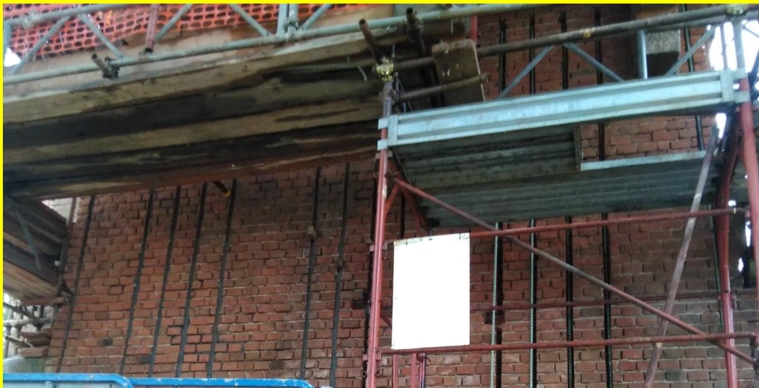
FIGURE 7: Piers were reinforced for bending using GFRP rods for out of plane and in plane bending
