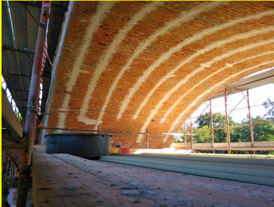
FIGURE 5: The reinforcement operations are finished, sleeves are painted to hide the reinforcement
