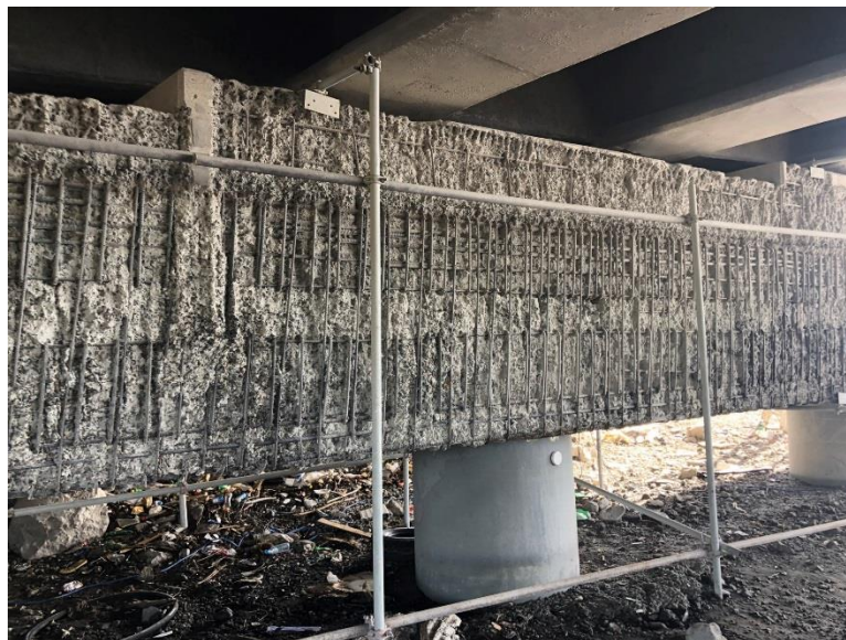
FIGURE 8: Bent cap after cover removal
