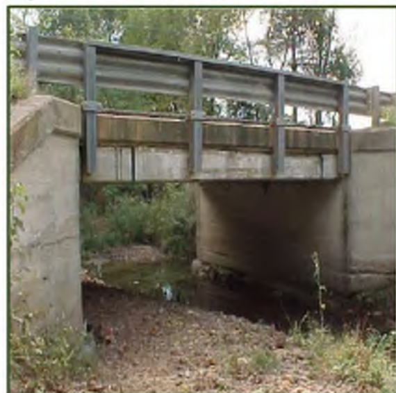
First Bridge Strengthened In Missouri: Year 1998 Bridge G270, Iron County, Missouri. Repair Technique: Externally Bonded Manual Wet-Layup CFRP Sheets.
