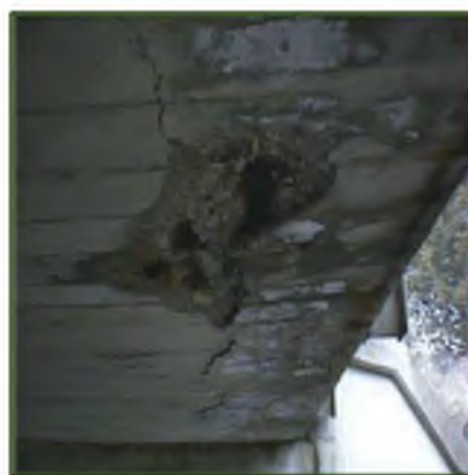
Concrete Distress Due to Corrosion Prior to Strengthening
