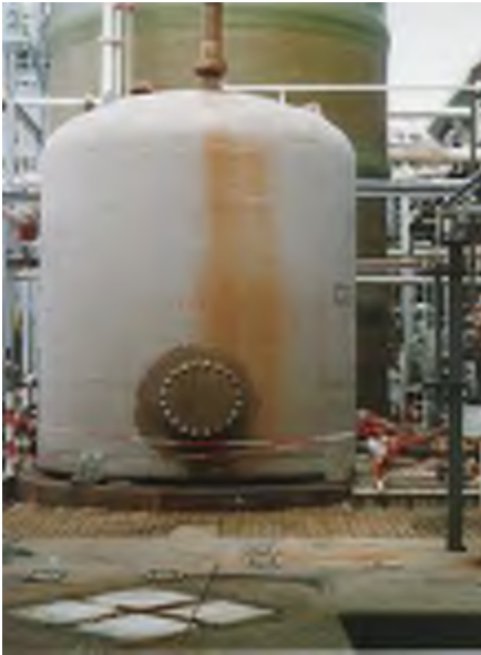
HCl Storage Tanks → 27 yrs
