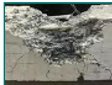
Concrete crushing (GG-4.7-G-100)
