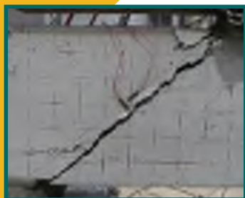
Diagonal strut tension failure (GG-1.8)
