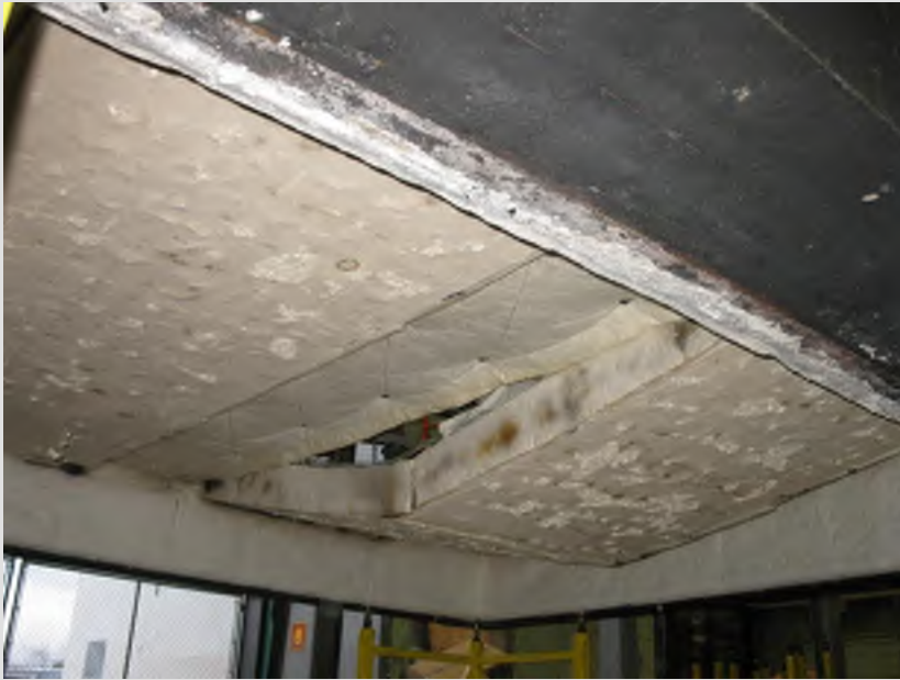
Failure of one of the slabs
