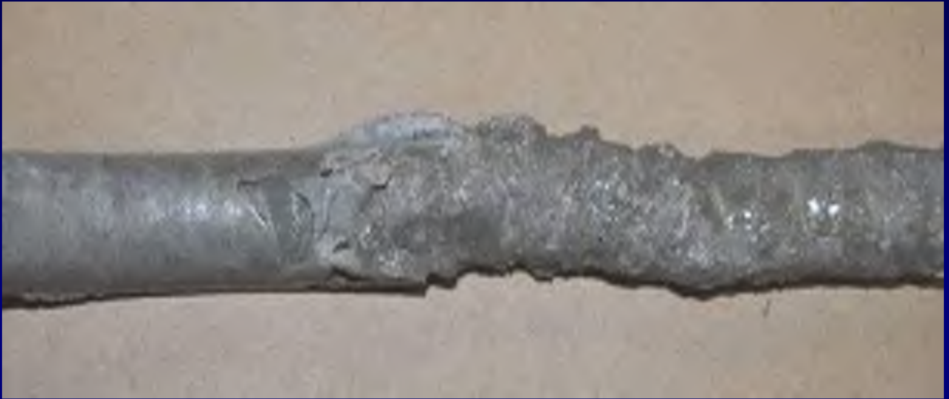
Unacceptable rebar with kink and rough finish
