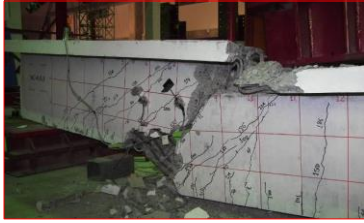
Shear Failure of SC-9.5-3 (CFRP @ d/3)
