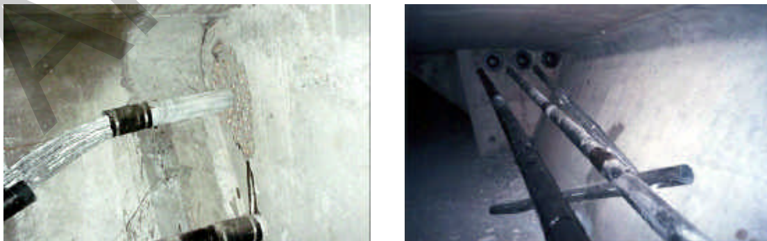
Figure 3.2 – Tendon 57-1: failure at Expansion Joint Diaphragm (left), View towards Pier Segment Diaphragm (right)
