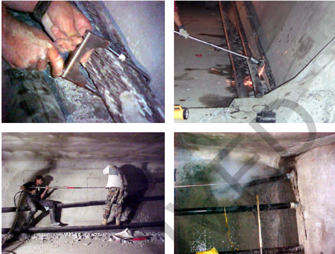
Figure 4.1 – Details of the Removal of External Tendons (Clockwise from upper left: clamping strands, cutting cable, hydro-blasting at pier segment diaphragm, and hydro-blasting operator)
