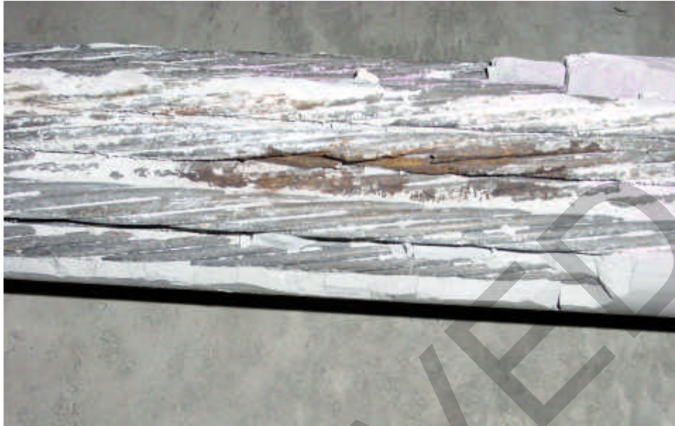
Figure 2.8 – Visual Inspection of Tendon 40-2 with corrosion in the free length of tendon.
