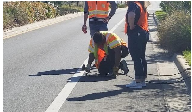
Figure 13: City of Tallahassee team installing the second bicycle counter along eastbound bicycle lane.
