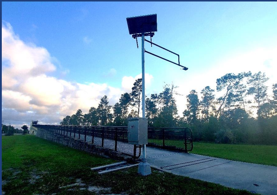
Q-Free Overhead passive infrared with piezo strips
