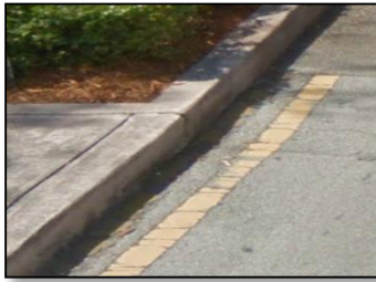
0 – Raised Curb (no shoulder or width exists)
