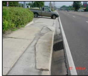
Curb inlet without manhole
