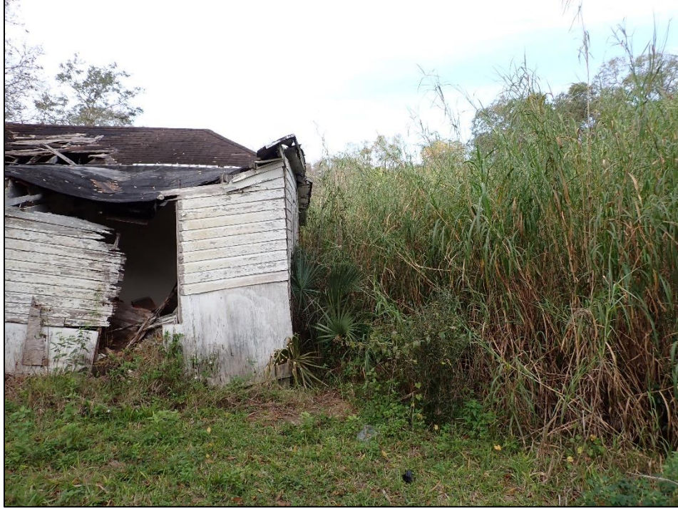
Figure 31: East End of Proposed Pond 1C, showing Dense Foliage and Dilapidated Structure, facing West
