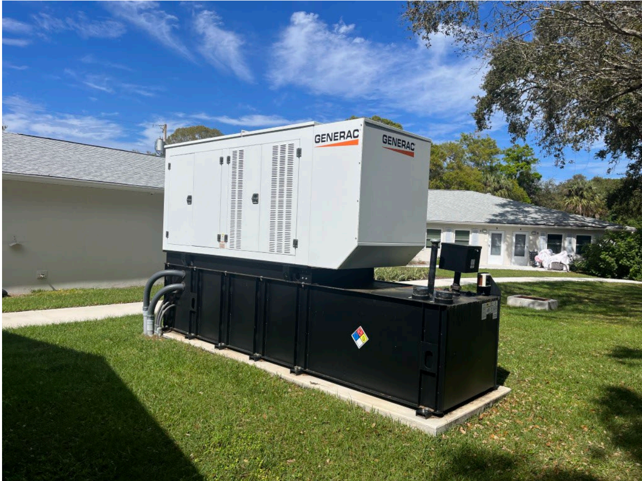
Photo 7. Map ID #7. Orange Blossom Village. This residential community has an emergency power generator with belly-mounted AST. Photo date 2/13/2024. View to north.
