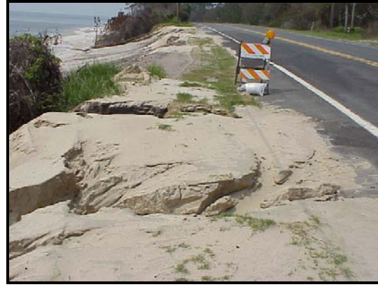
Sheet and gully erosion along shoulder, August 2005
