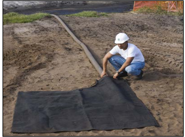
Gravity Bag Filter (Source: http://www.spillcontainment.com )
