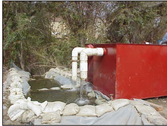
Dewatering Tank (Source: http://www.dot.ca.gov )
