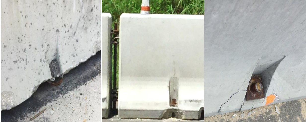
Figure 10: Examples of Unacceptable Type K or Proprietary Concrete Barrier with broken concrete or shear cracking at the anchor slot – From left to right: Concrete has completely broken away at the anchor slot due to shear cracking; Broken concrete at the anchor slot due to shear cracking; Broken concrete at the anchor slot due to shear cracking.
