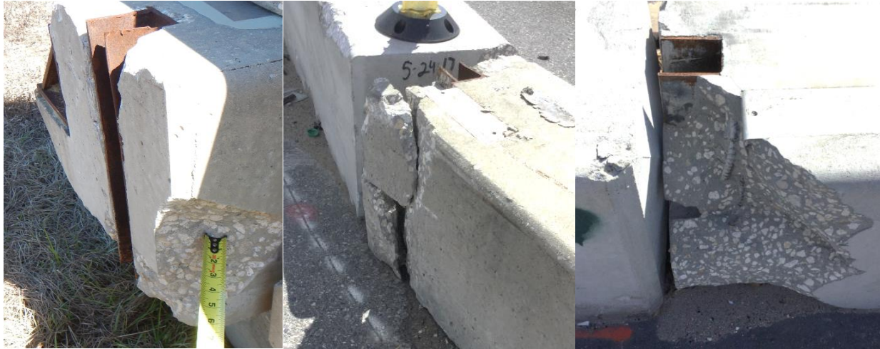
Figure 6: Examples of Unacceptable Low-Profile Concrete Barrier – From left to right: Barrier with spall greater than 1.5 inches; Barrier with cracked and broken concrete that could easily be dislodged resulting in conditions 1 or 2 above; Barrier with damage to a connection assembly and spalling greater than 1.5 inches in depth with exposed rebar.
