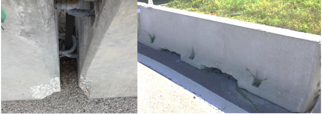
Figure 5: Examples of Acceptable Type K or Proprietary Concrete Barrier with spalls of 1.5 inches or less
