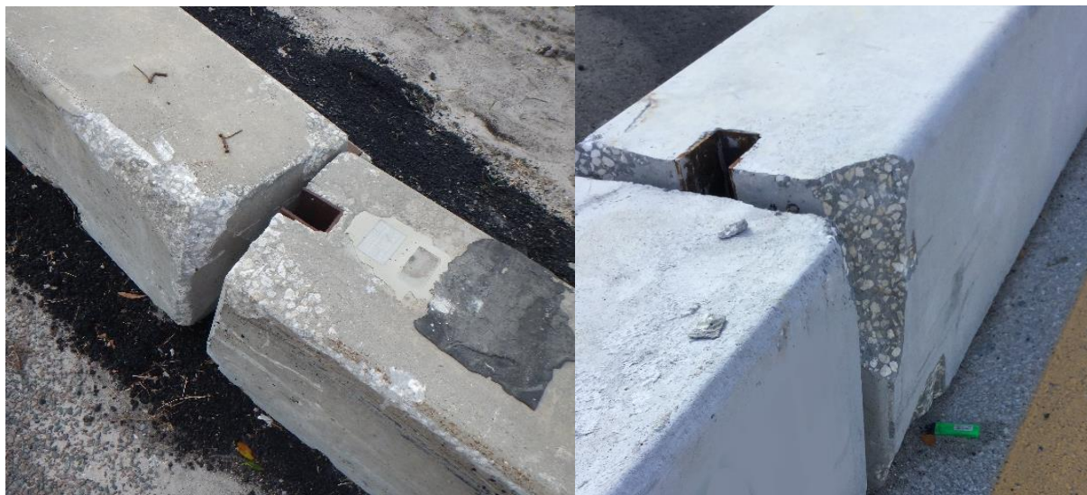
Figure 2: Acceptable Low-Profile Concrete Barrier with spalls of 1.5 inches or less
