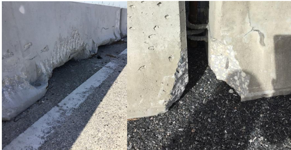
Figure 9: Examples of Unacceptable Type K or Proprietary Concrete Barrier with spalls greater than 1.5 inches– From left to right: Barrier has spalls greater than 1.5 inches in depth; Barriers have spalls greater than 1.5 inches in depth and the righthand unit has exposed rebar.
