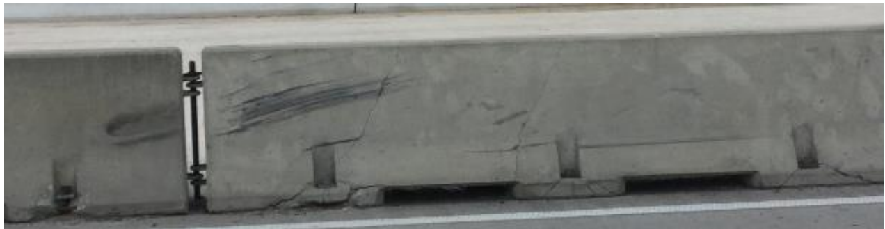
Figure 7: Example of Unacceptable Type K or Proprietary Concrete Barrier – Barrier has multiple cracks that extend through the entire cross-section and broken concrete with shear cracking around the anchor slots.
