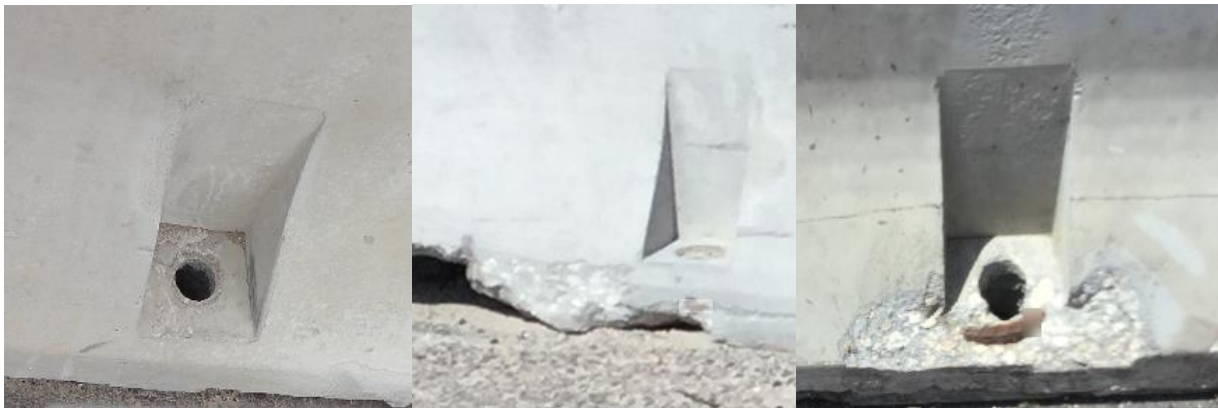
Figure 4: Acceptable Type K or Proprietary Concrete Barrier Anchor Slots – From left to right: Undamaged anchor slot; Anchor slot with spalled concrete less than 1.5 inches in depth; Anchor slot with spalled concrete less than 1.5 inches in depth and exposed rebar
