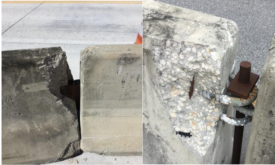
Figure 8: Examples of Unacceptable Type K or Proprietary Concrete Barrier with connection assembly damage – From left to right: Barrier has damage to unit-to-unit connection assembly and spalls greater than 1.5 inches in depth; Barrier has damage to unit-to-unit connection assembly, spalls greater than 1.5 inches in depth, and exposed rebar.
