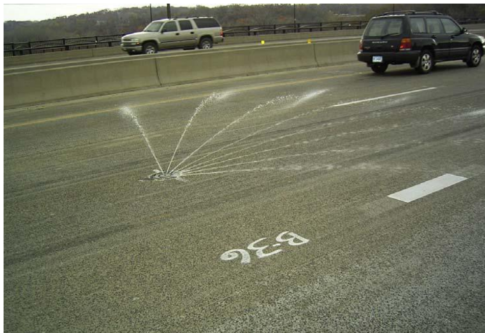
FIGURE 45 Anti-icing system on a bridge.
