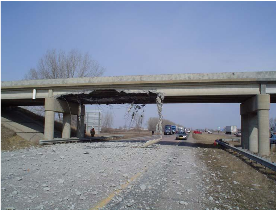
FIGURE 24 Interstate closure after an impact with a bridge.
