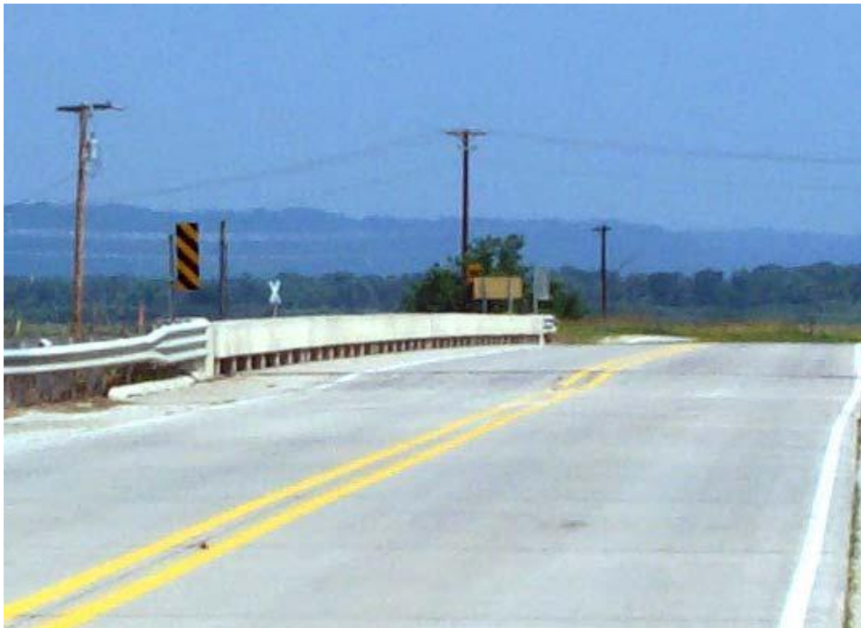
FIGURE 46 Bridge rail and guardrail transition in compliance with NCHRP Report 350 .
