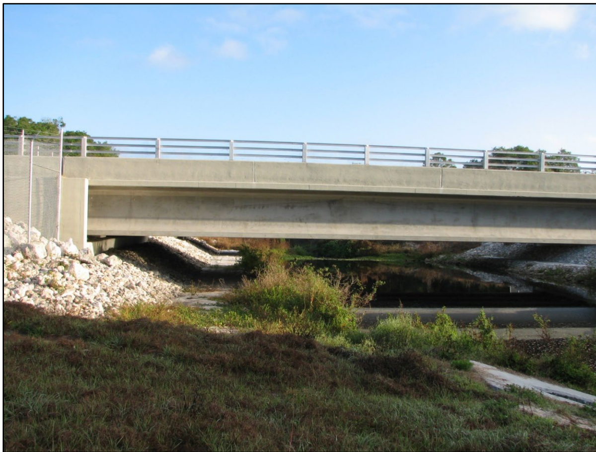
Figure 17 – 1 Bridge with Shelves for Wildlife
