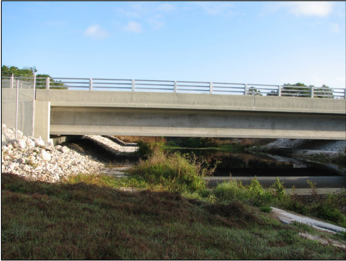
Figure 17 – 1 Bridge with Shelves for Wildlife
