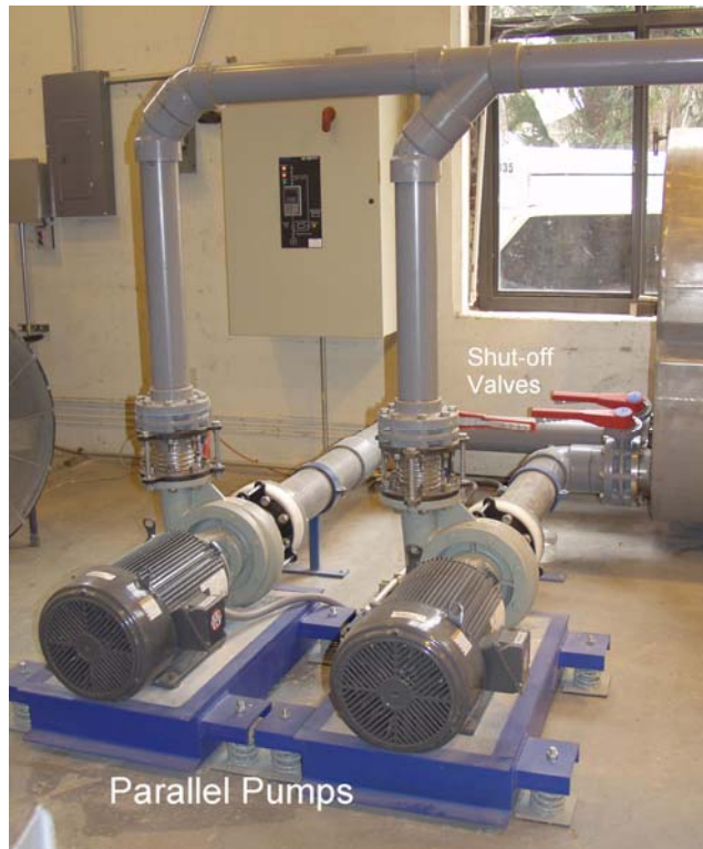
Figure A-2 Photograph of the SERF pumps and valves.
