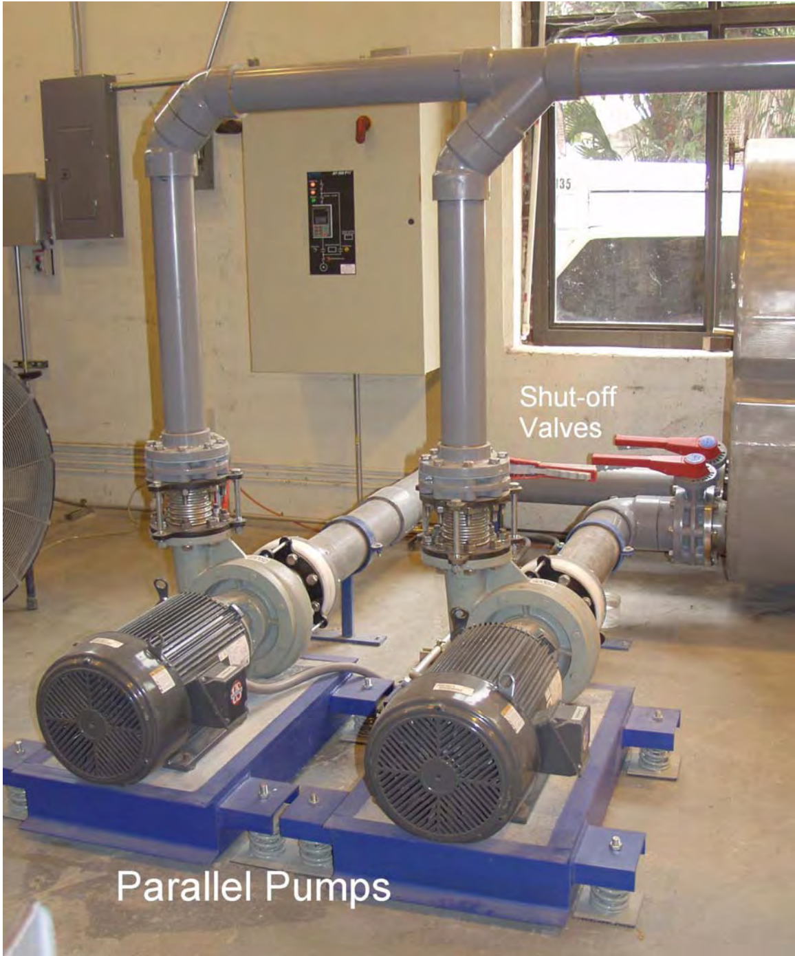
Figure IID - 2. The Pumps with Shut-Off Valves, Plumbing, and Pumps on the Inertial Bases.
