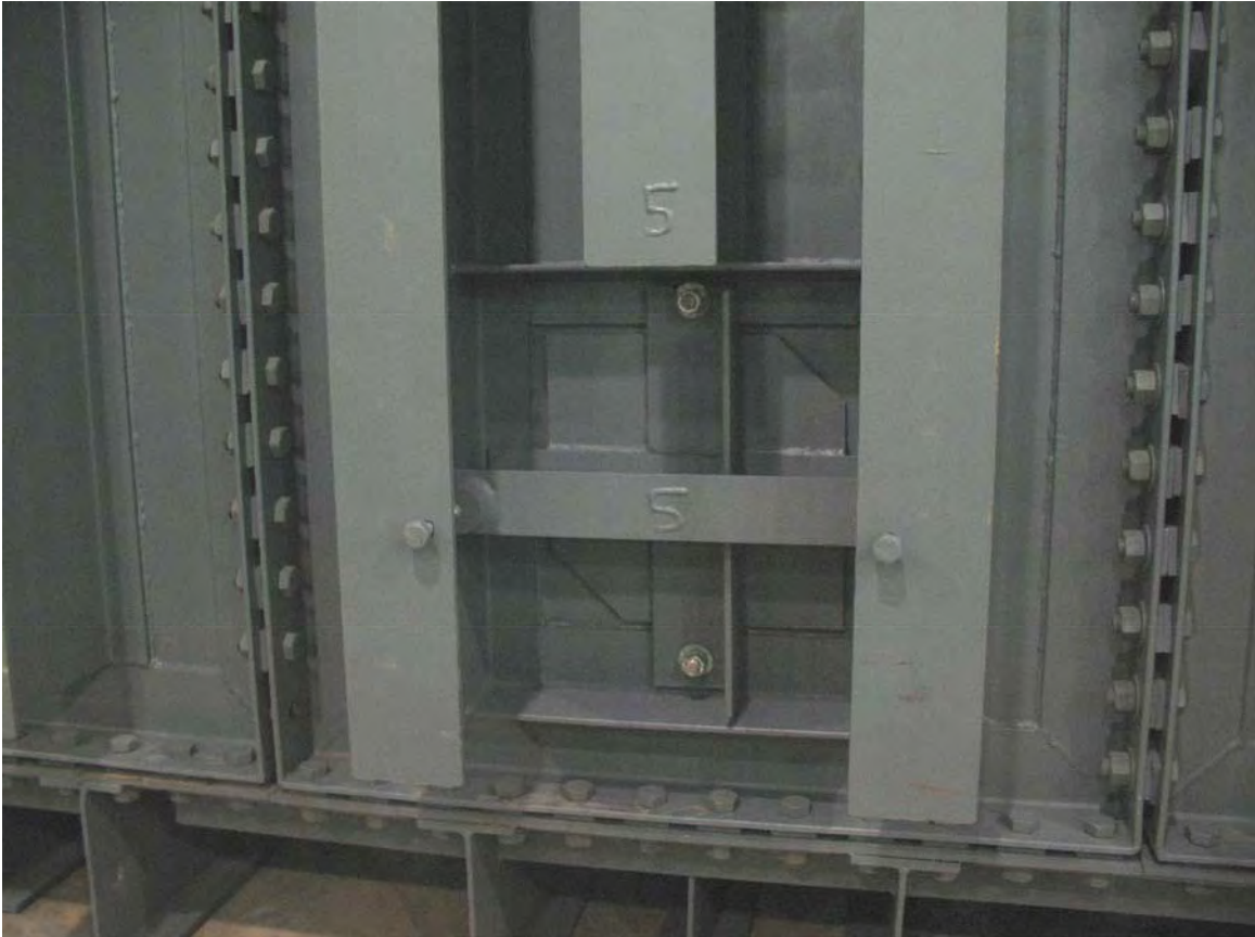
e) Pipe Access hole and cover
