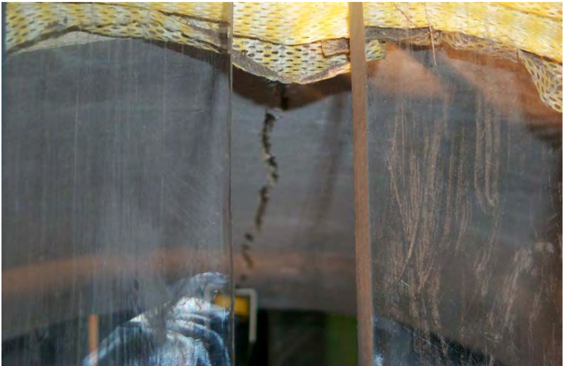
Figure A-2.10 Flexure crack at the crown of fiber reinforced concrete pipe.
