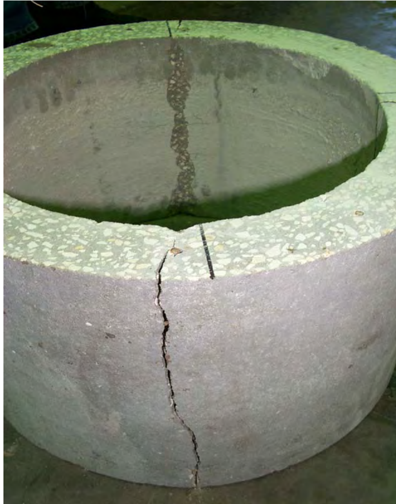
Figure A-3.3 Standard reinforced concrete pipe section cracked.
