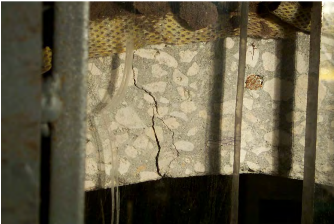
Figure A-2.11 Reinforced concrete pipe cracking at the crown.
