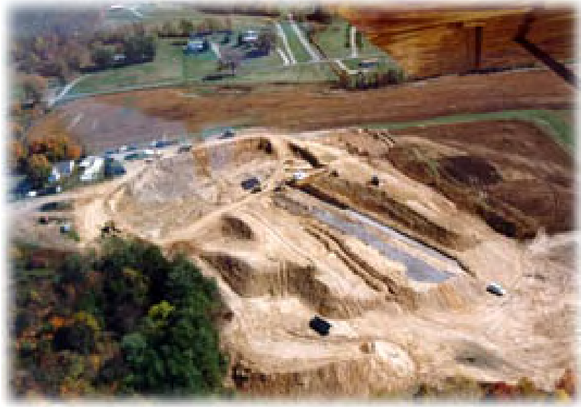
Figure A-2.4 The Center for Pipes and Underground Structures test facility at Ohio University. (Courtesy of James Hardie Pipe, Inc.)
