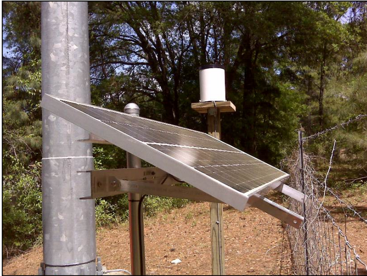
Solar panel and rain gage
