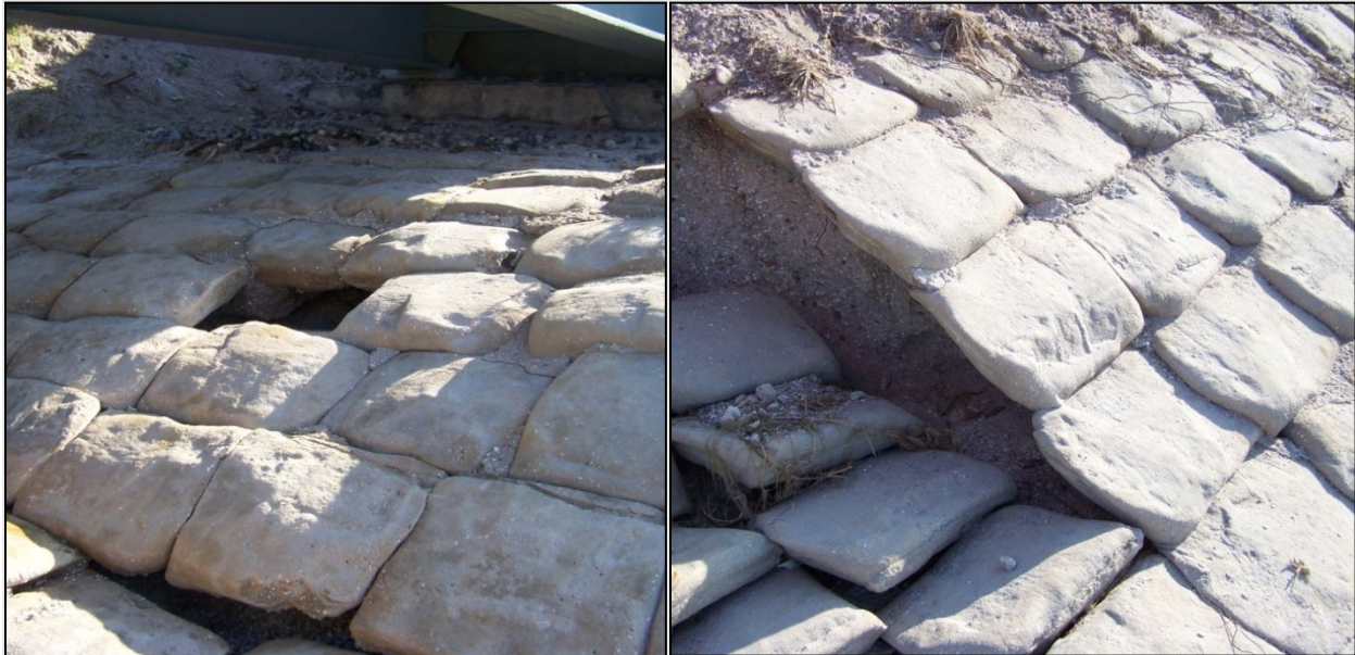
Figure 5.5-11: Damage to Sand-Cement Grouted Riprap Abutment Protection
