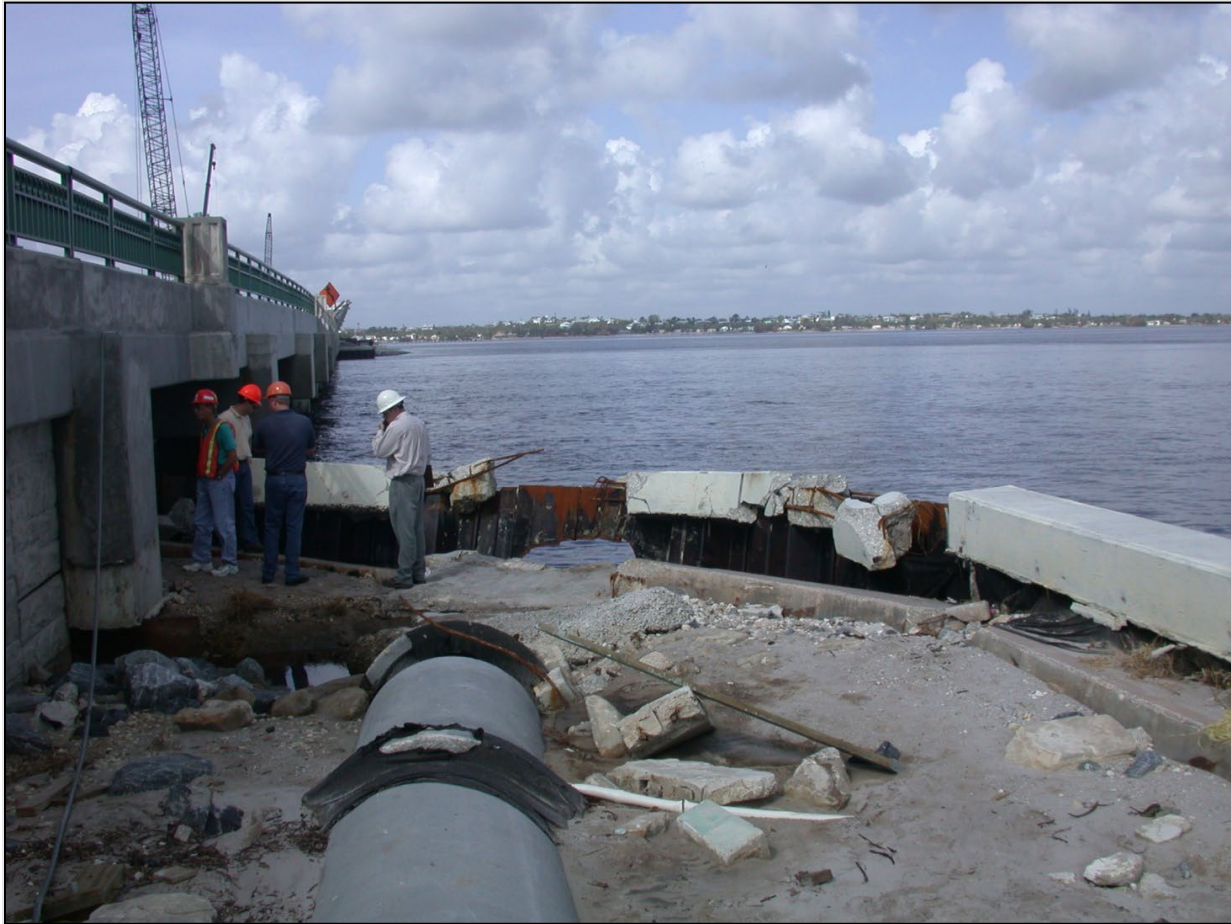
Figure 5.5-17: Seawall Failure Following Hurricane Frances (2004)
