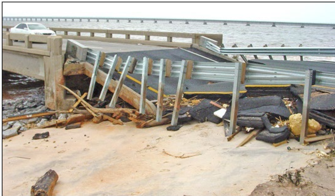
Figure 5.5-6: East Approach to the I-10 WB Bridge over Escambia Bay After Hurricane Ivan (2004)
