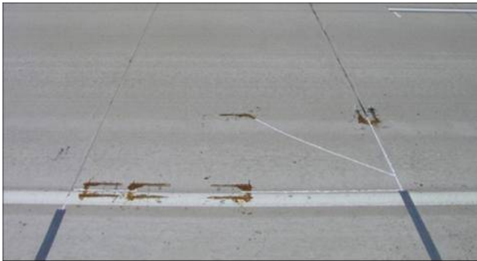
Figure 2-5. Surface strain gauges on surface of whitetopping.
