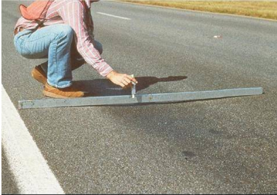
Figure 3-7. Photograph of HMA permanent deformation.
