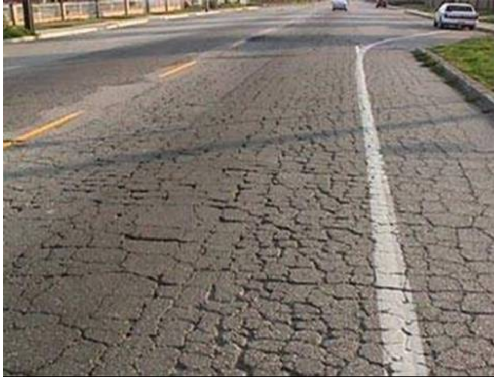
Figure 3-2. Photograph of fatigue cracking.
