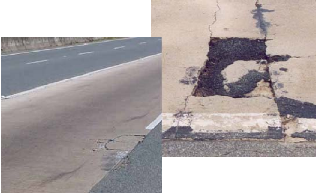
Figure 3-14. Photograph of CRCP punchouts.
