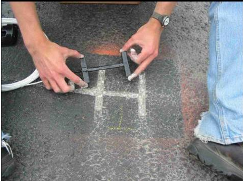
Figure 2-1. Typical HMA horizontal strain sensor (H-sensor).
