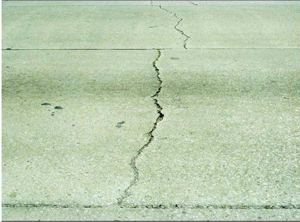
Figure 3-9. Photograph of JPCP transverse cracking.
