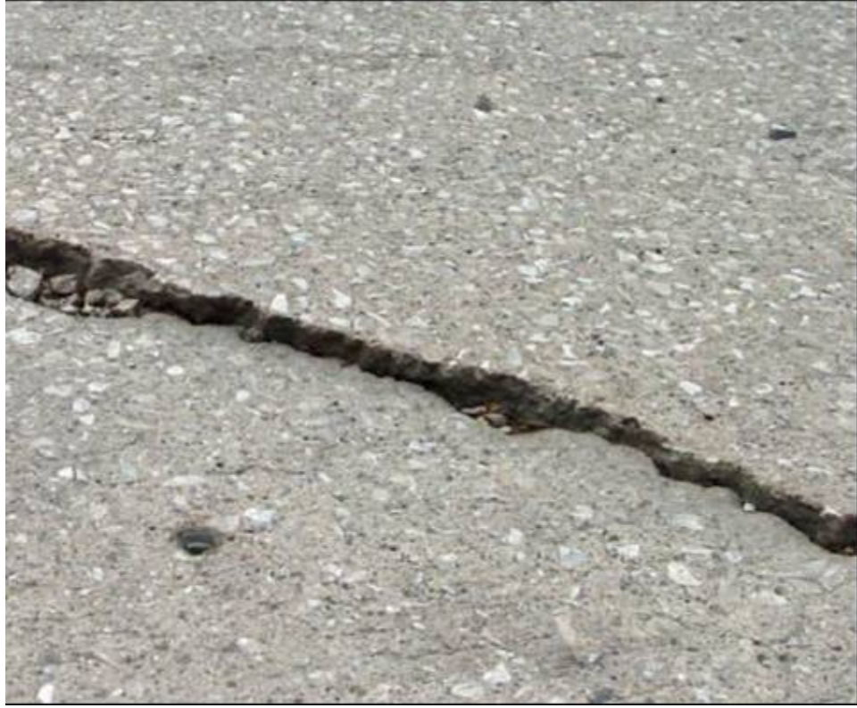
Figure 3-12. Photograph of JPCP faulting.
