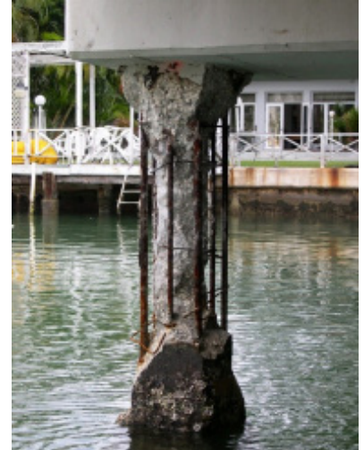
Concrete corrosion, as shown here, impacts the service life of critical transportation facilities like bridges.
