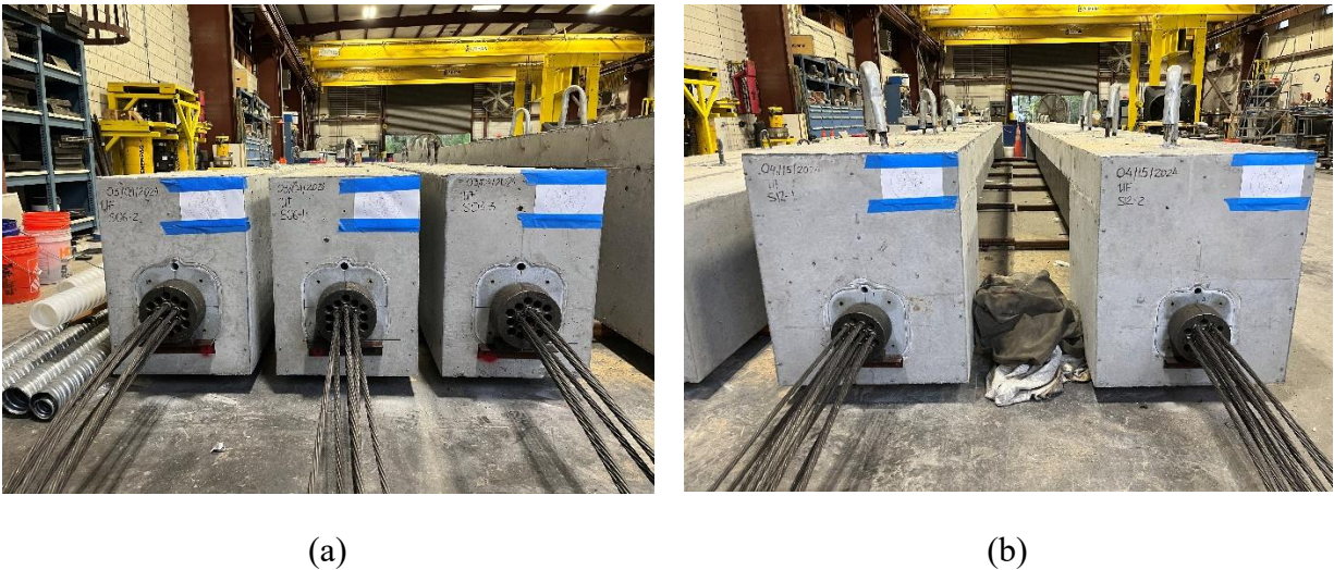
Figure 6.10. Prestressing strands projecting out of the wedge plate at live ends: (a) S06; (b) S12 beams.
