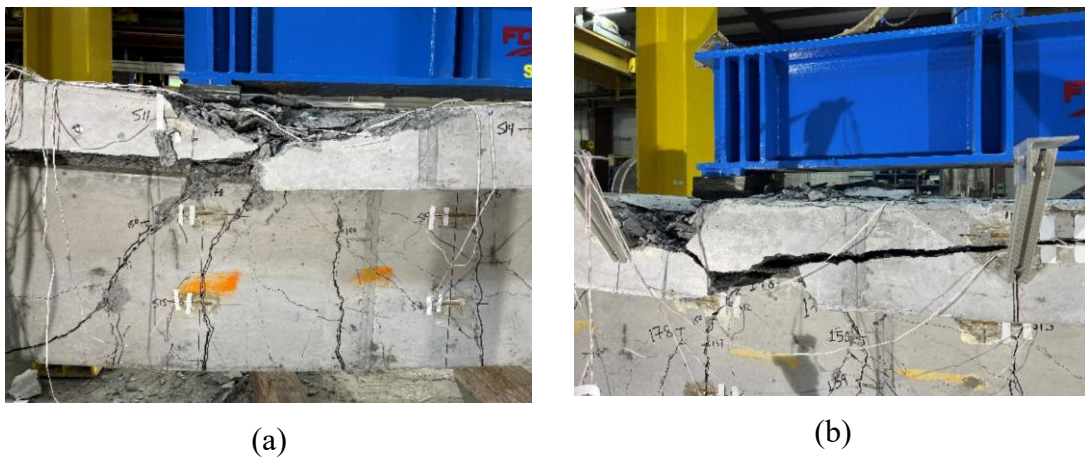
Figure 9.16. Crushing of concrete at the compression flange: (a) D19-M-U; (b) D19-M-T.
