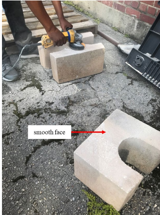
Figure 3-25. Grinding the lug off the tops of the Vertica Straight Face blocks.
