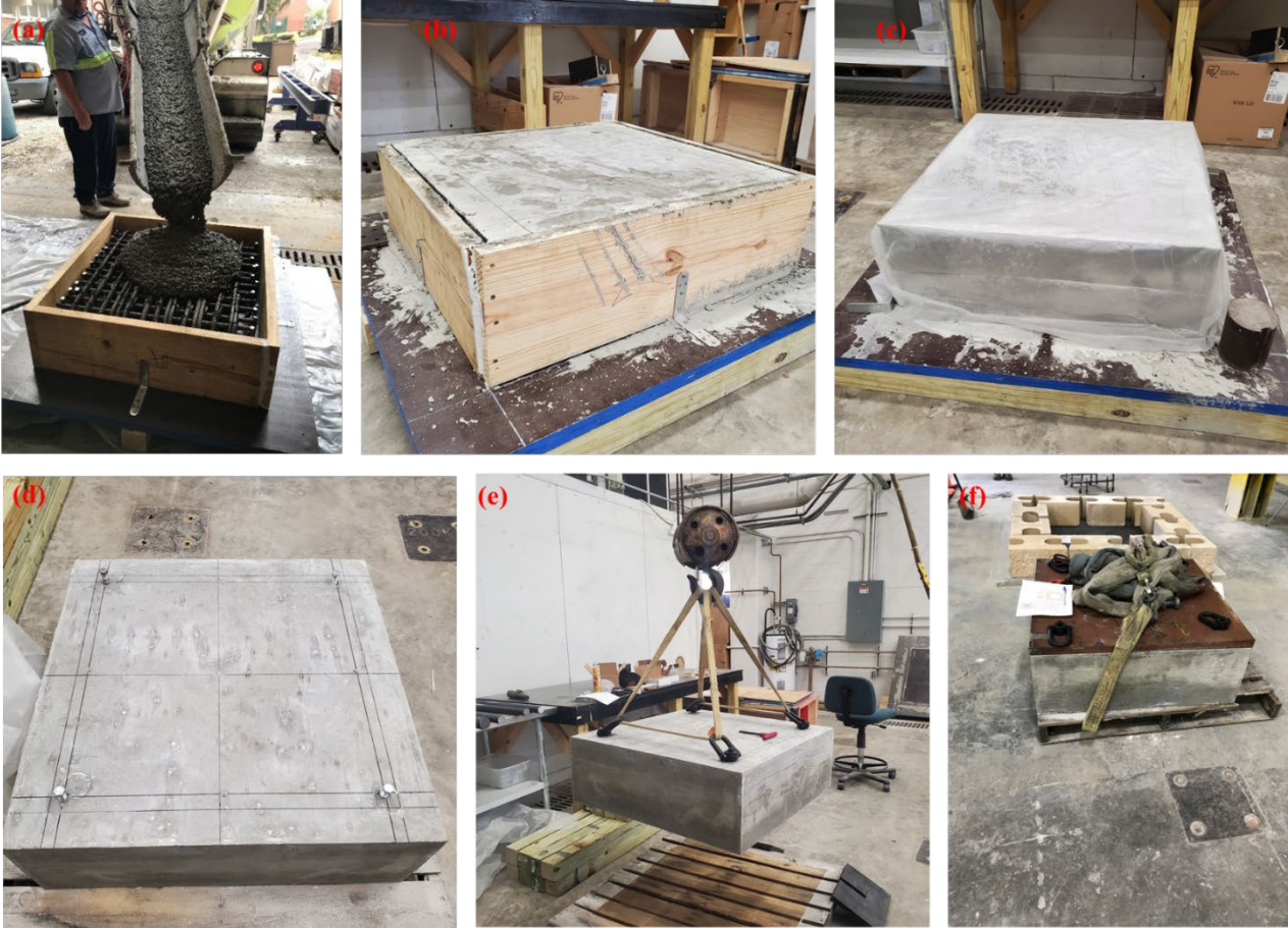
Figure 3-26. Casting of a concrete footing. (a) Pouring of concrete (b & c) Curing of concrete (d) Installation of anchor bolts (e) Testing the installed anchor by lifting (f) Finished footing with steel plate.
