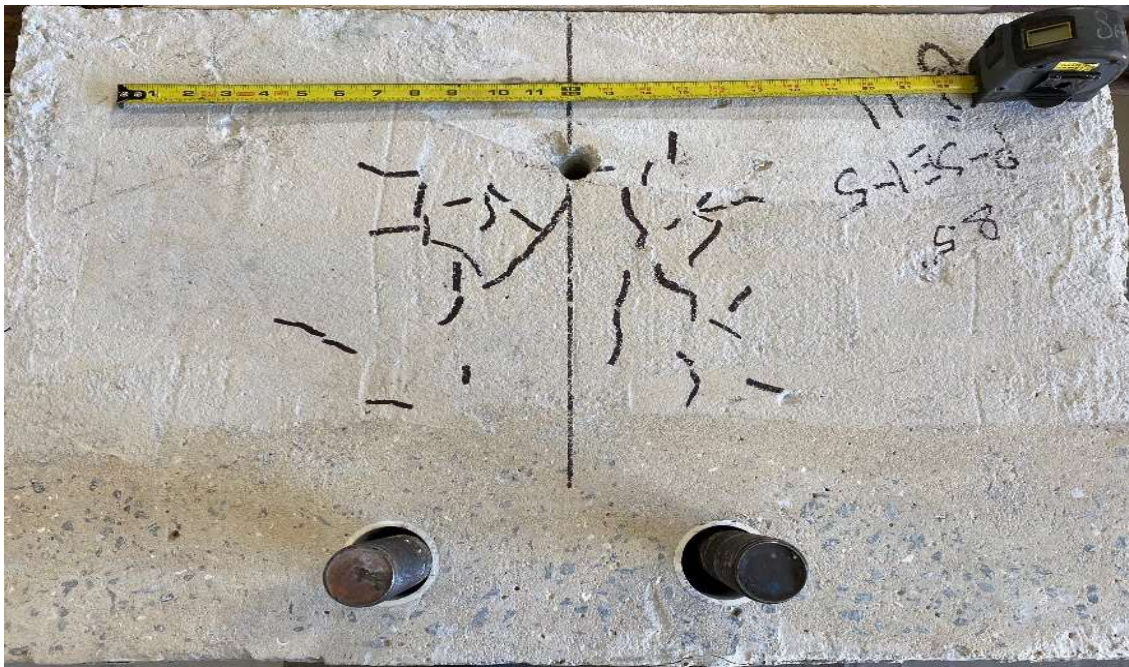
Figure A-14: P-SE1-5 specimen concrete after loading
