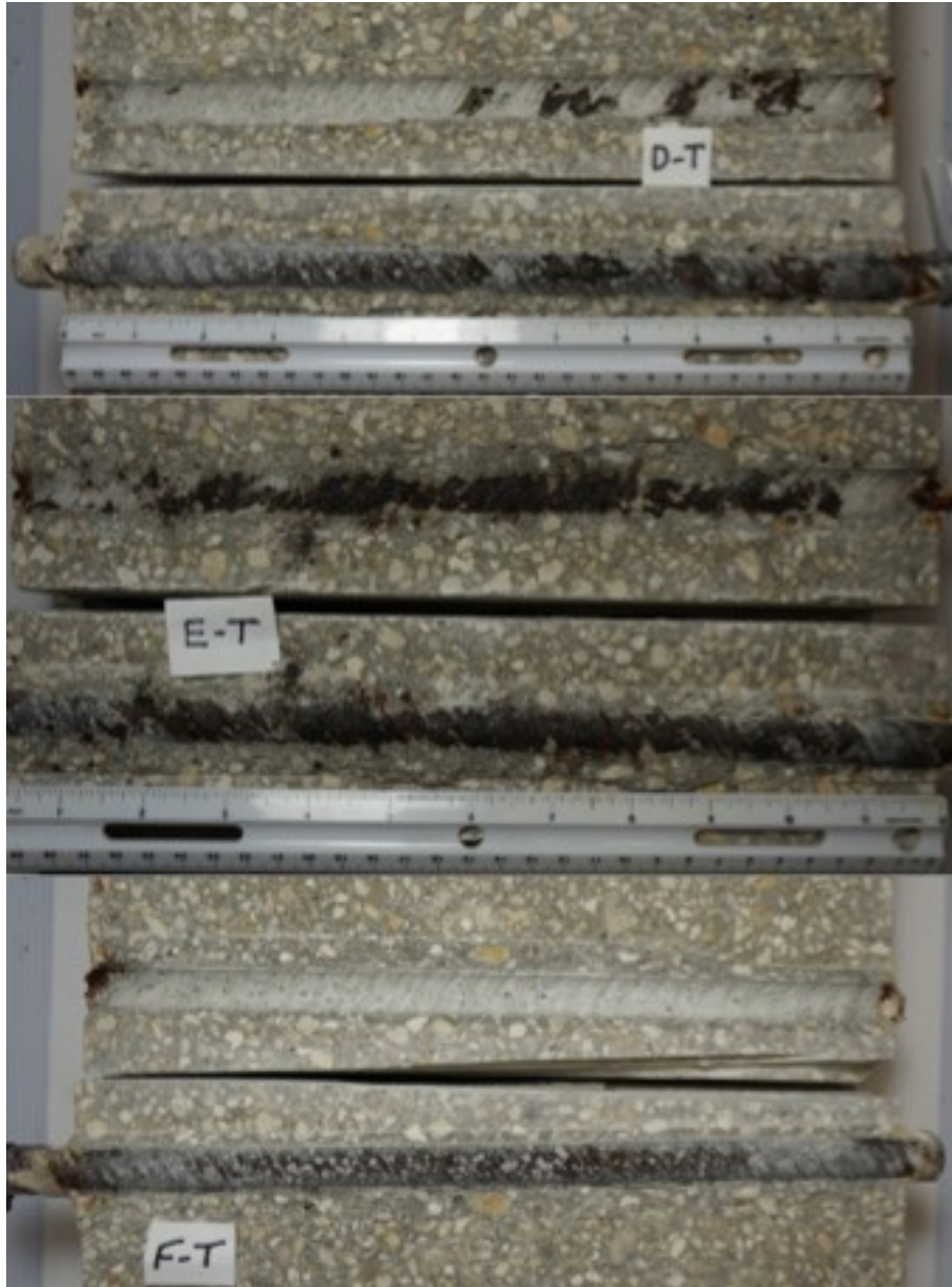
Figure 7-3. 4-CCRV-3CR12-2 bottom row, top-facing rebars and concrete rebar traces.
