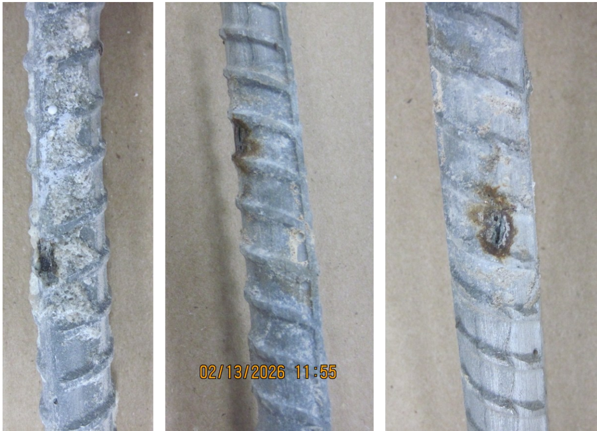
Figure 8-22. Close up corrosion spots on rebar 1 of sample BENT-STD3-304-C.
