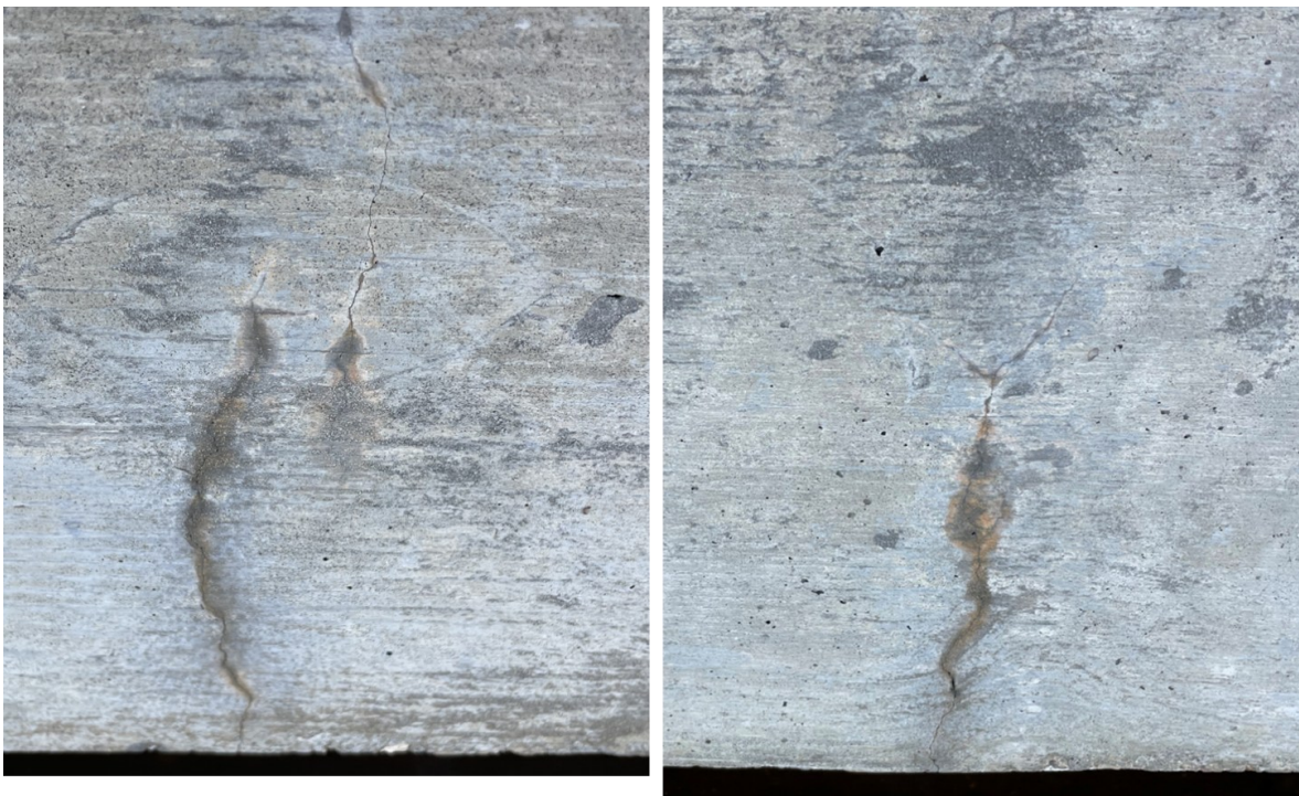
Figure 6-4. Close-up of two of the cracks (moisture allows for observation).
