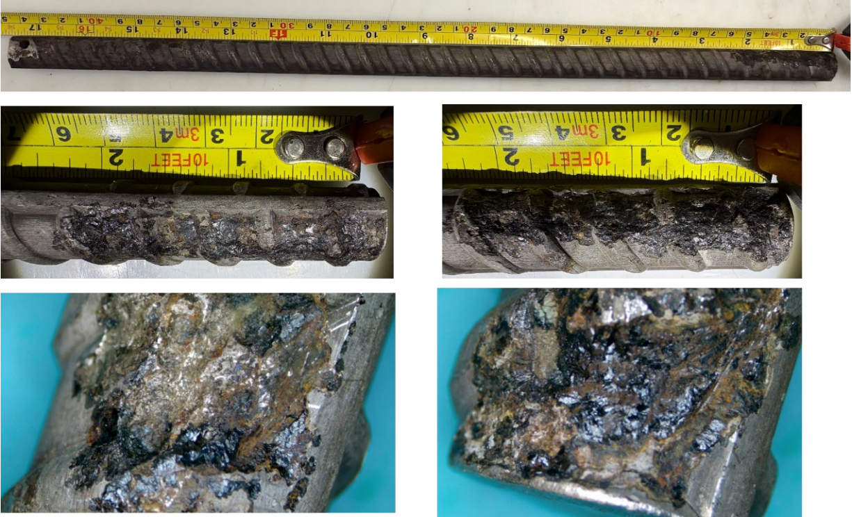
Figure 8-51. STD3-MMFX-B - full length of rebar 2 and notable areas of corrosion damage.
