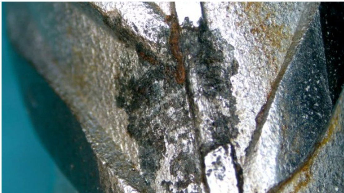
Figure 8-40. Corrosion spot observed on rebar 2 of STD3-2101-B.
