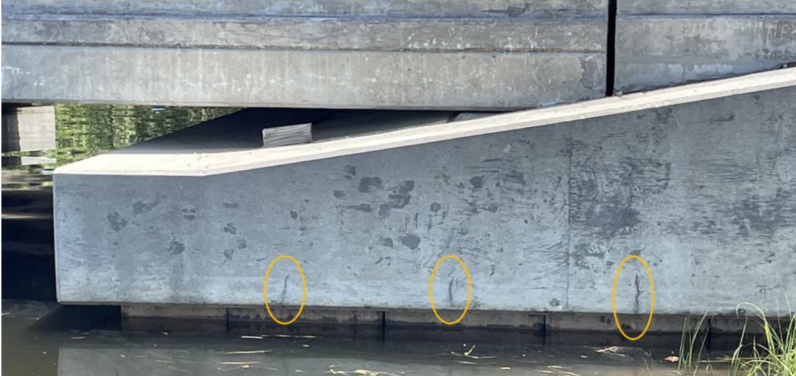
Figure 6-3. South side of the bridge, showing several cracks (moisture allows for observation).
