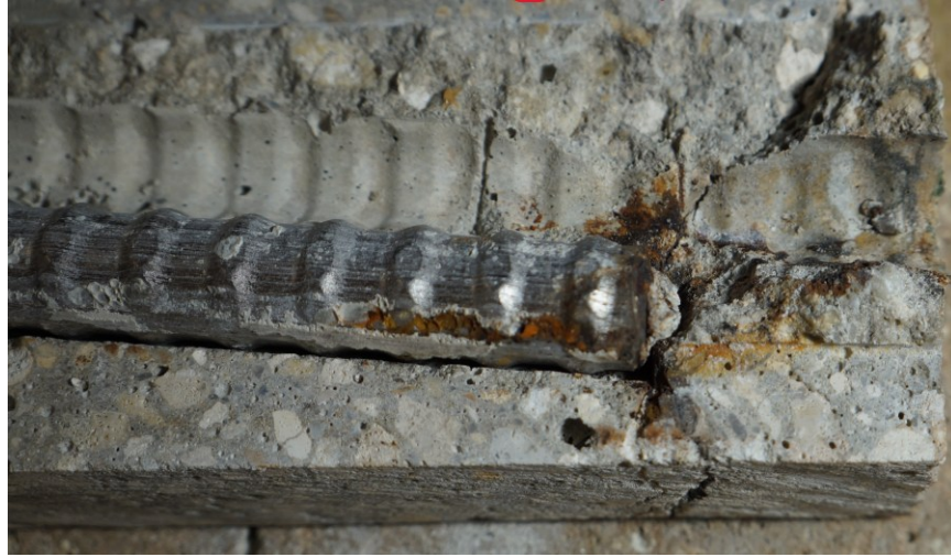
Figure 7-34. Concrete crack caused by corrosion from rebar C1.
