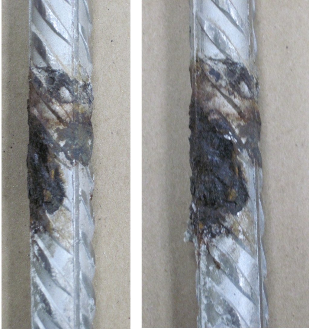
Figure 8-18. Close up of corrosion spot on rebar 3 of sample STD3-2101-B at multiple angles.
