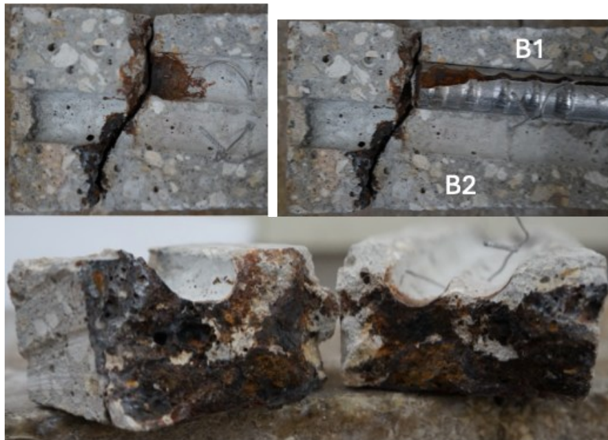
Figure 7-32. Concrete fracture caused by corrosion from rebar B1.
