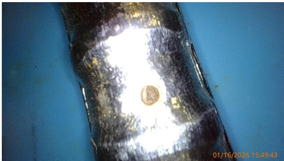
Figure 7-53. Hole 4 on bottom side of rebar C of sample BCCD-CT2-1.
