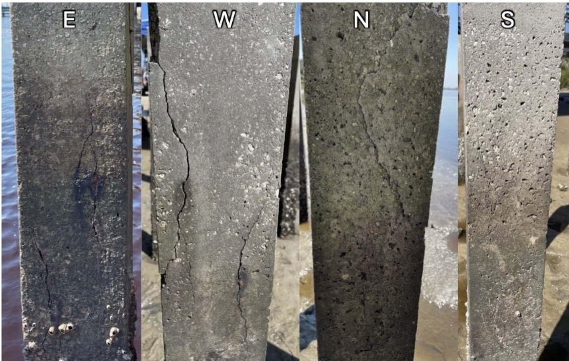
Figure 5-9. Picture showing cracks on the surface of each face of column 2101-C.
