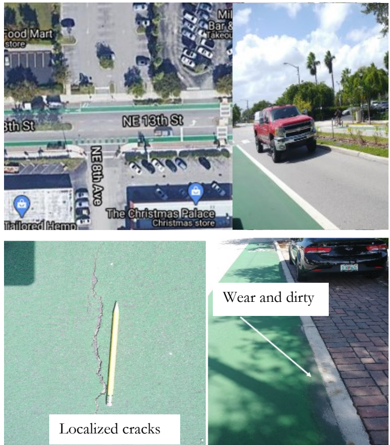
Figure A-22. Site 56-Location and Distresses.
