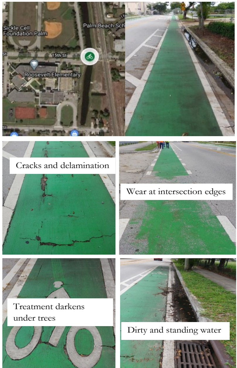
Figure A-15. Site 17-Location and Distresses.
