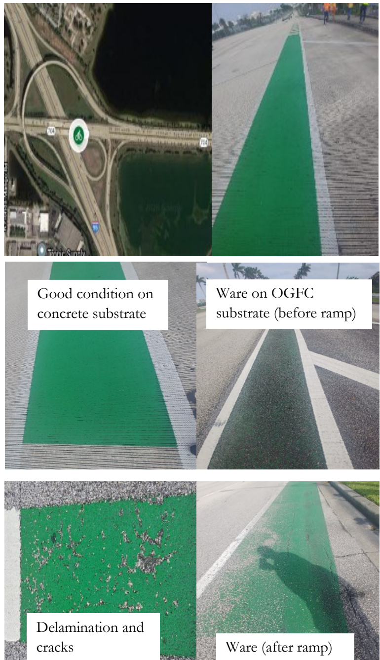
Figure A-16. Site 18-Location and Distresses.
