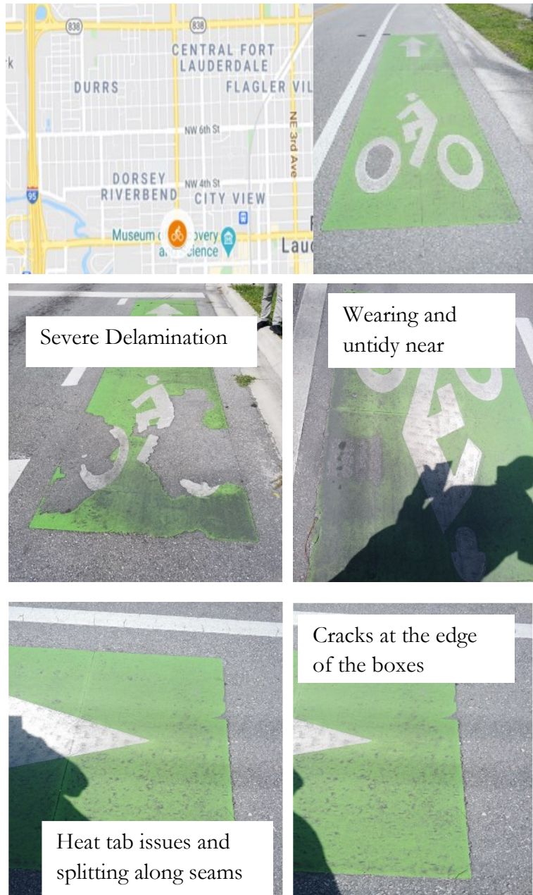
Figure A-6. Site 24-Location and Distresses.
