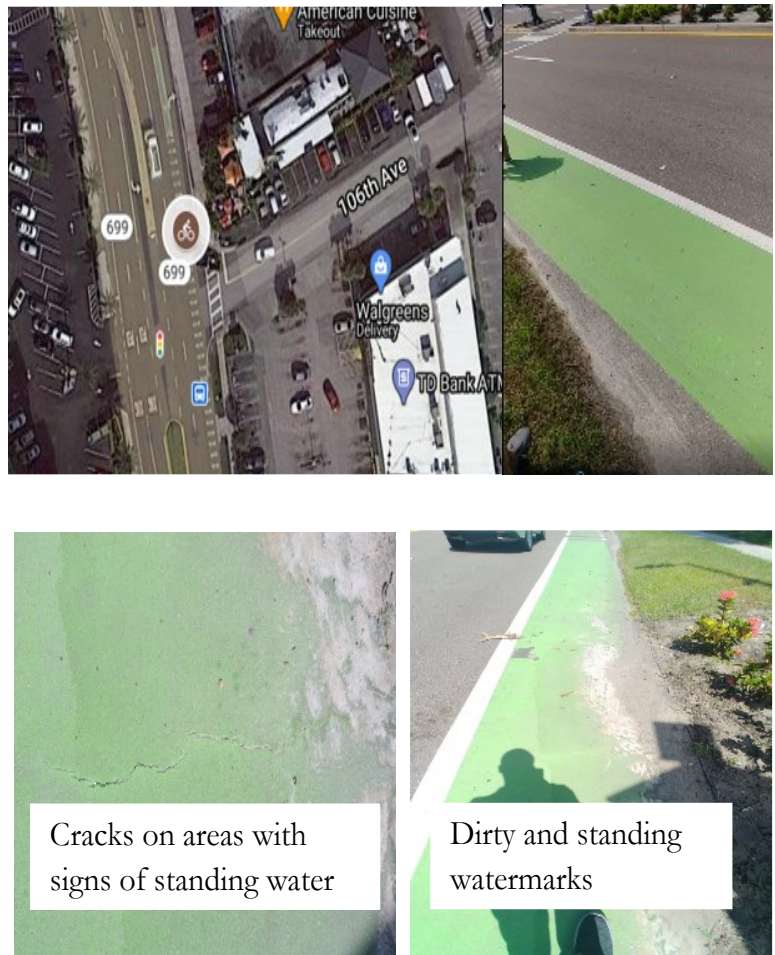
Figure A-9. Site 3-Location and Distresses.
