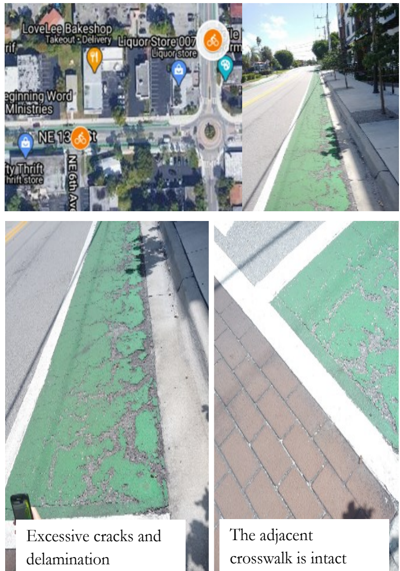
Figure A-21. Site 23 and 55-Location and Distresses.
