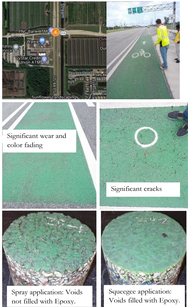
Figure A-19. Site 20-Location and Distresses.
