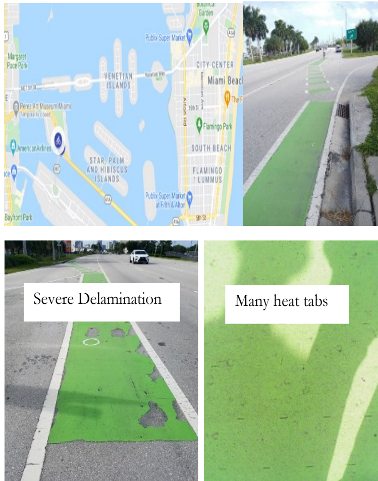
Figure A-7. Site 28 and 29-Location and Distresses.
