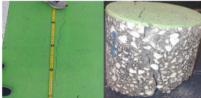
Figure 3-7. Core Showing Extent of a Crack Observed in the Field.
