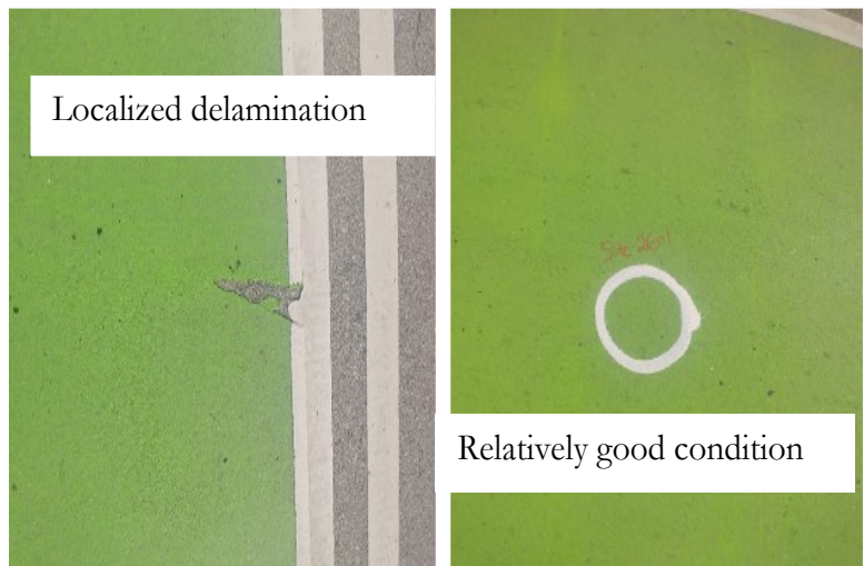
Figure A-4. Site 26-Location and Distresses.
