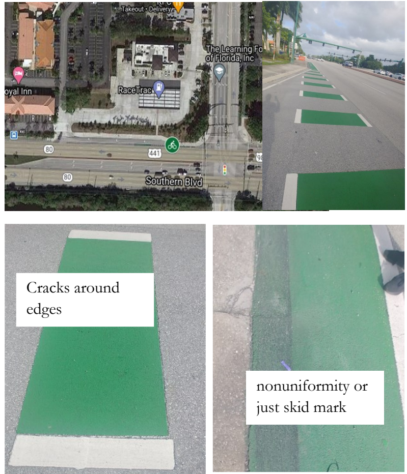
Figure A-17. Site 34-Location and Distresses.
