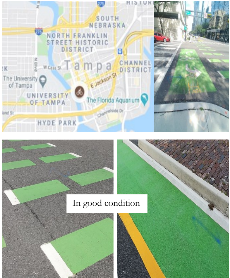
Figure A-12. Site 2-Location and Distresses.
