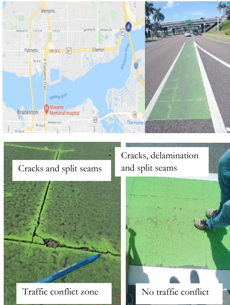
Figure A-8. Site 1-Location and Distresses.
