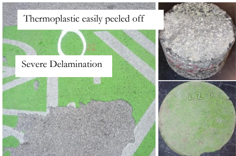
Figure A-5. Site 22-Location and Distresses.
