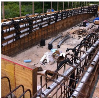
(c) Corrugated metal and plastic ducts being installed within the girder wall
