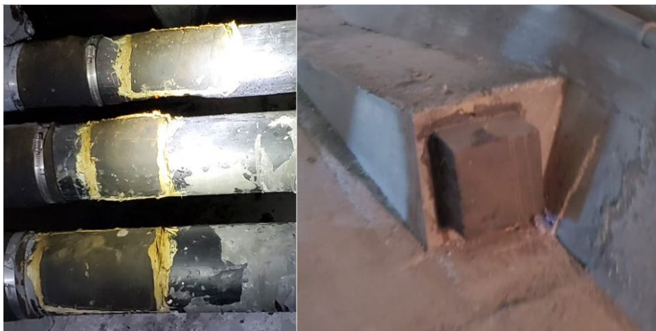
Figure 8. External ducts that were previously targeted for invasive inspection (Broadway Bridge) and concrete pourback for anchorage protection (Seabreeze Bridge).
