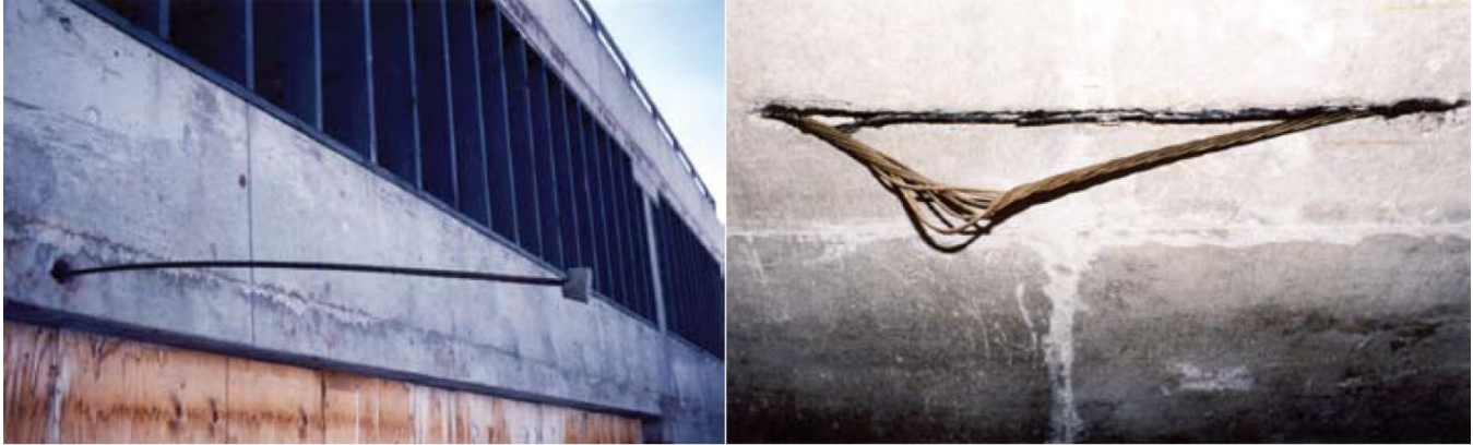
Figure 58. Erupted or ejected tendons from anchorage and slab soffit (Fallis et al. 45 )
