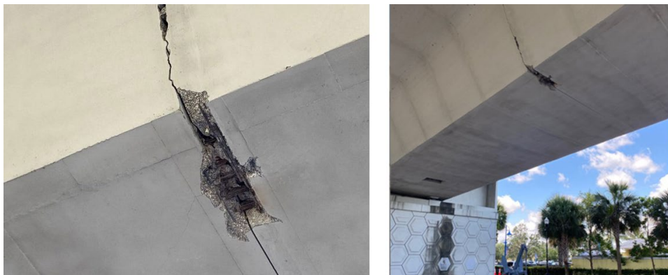
Figure 3. Localized corrosion damage for internal tendon on Roosevelt Bridge in Stuart, FL. (A) Concrete spalling and exposed tendons 8 and (B) location on bridge 9
