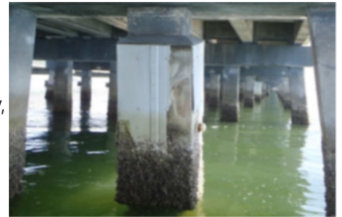
Sections of the fiberglass jacket installed to prevent corrosion have broken off of this pile.
