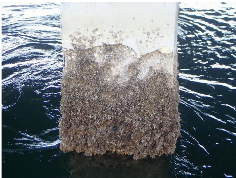
Figure 70. Missing portion of pile jacket (Pile 12-1)
