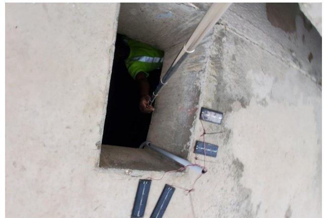
Figure 43. Overview of solar panels epoxied to the underside of the box girder (photograph provided by FDOT).
