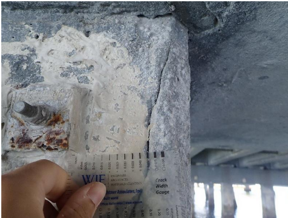
Figure 74. Cracking measured up to approximately 50 mil wide (Pile 44-5)
