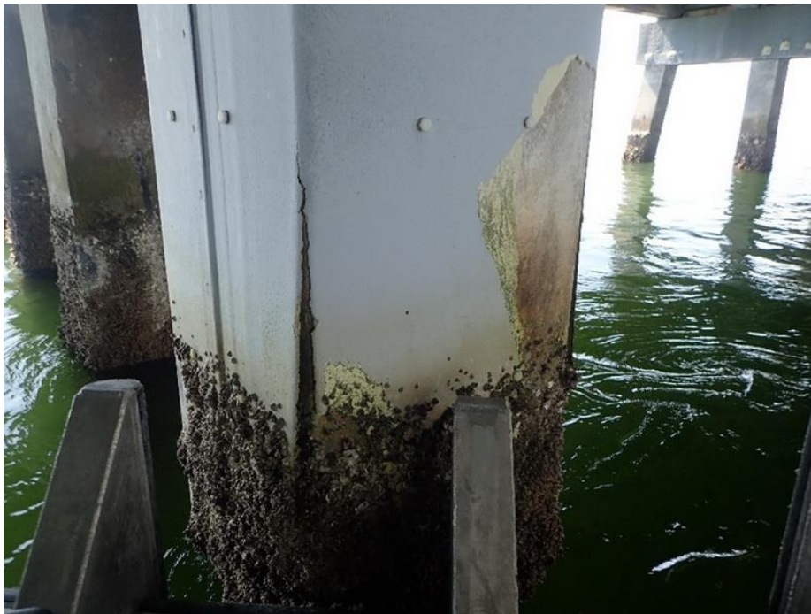
Figure 86. Significant distress of jacket (Pile 133-5)
