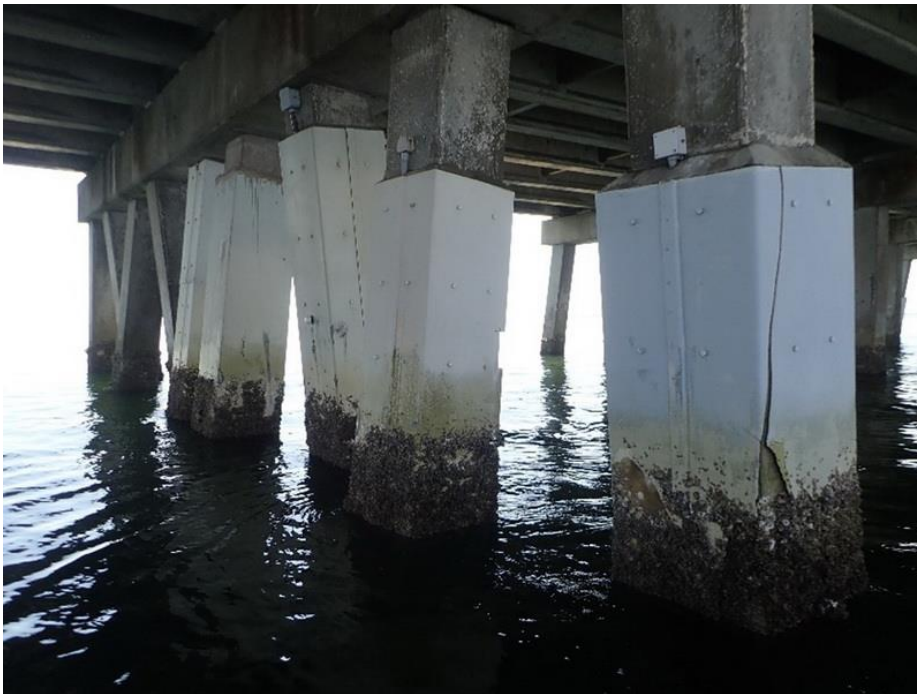
Figure 90. Vertical cracking of jacket (Pile 182-3)
