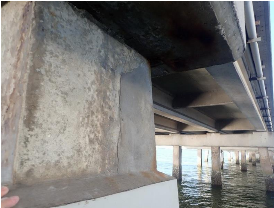
Figure 110. Cracking on repair of pile (Pile 104-1)
