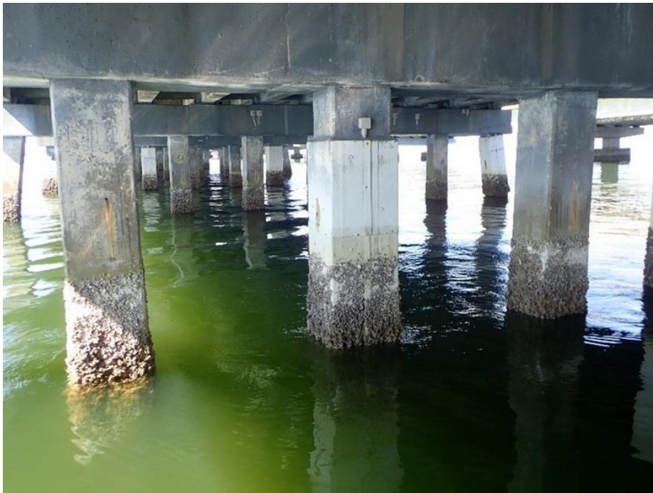
Figure 78. Overview photograph of apparent jacket extension on top (Pile 80-6)
