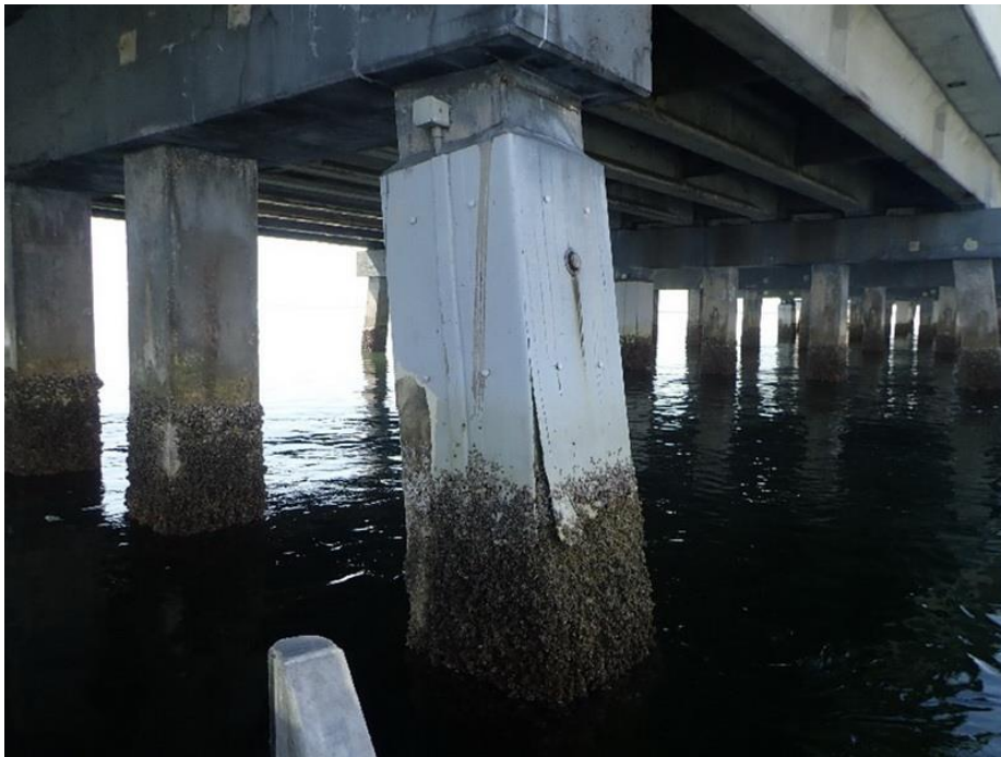
Figure 82. Significant distress of jacket (Pile 120-1)
