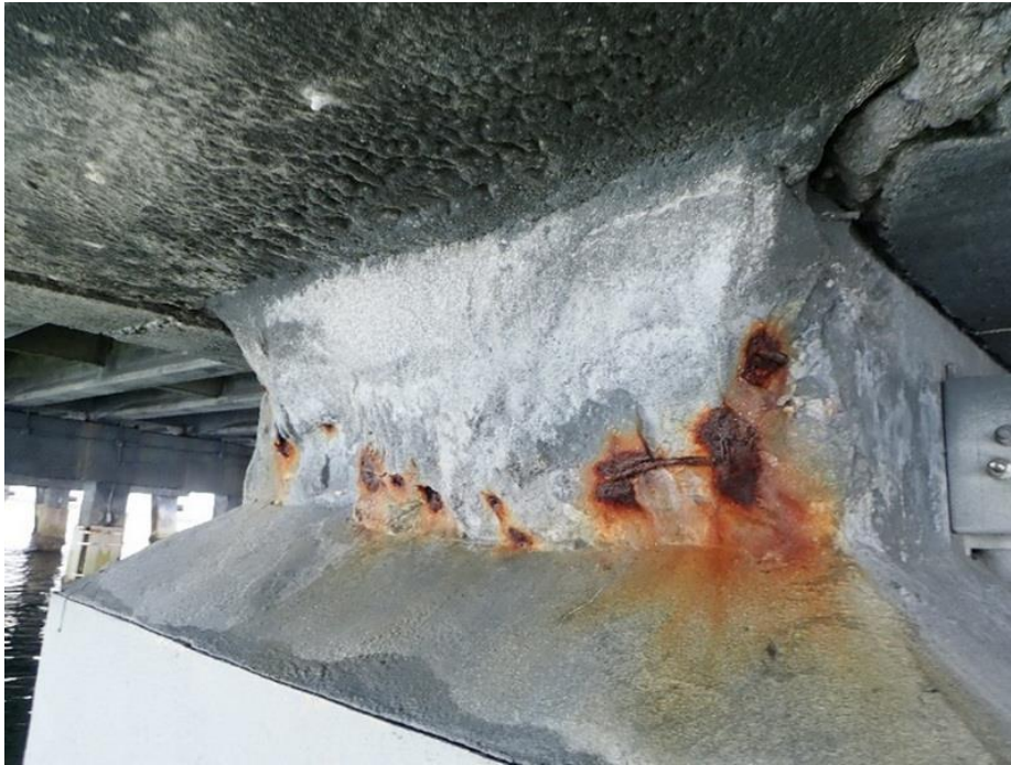
Figure 95. Repairs with corroded anchors on pile (Pile 214-6)
