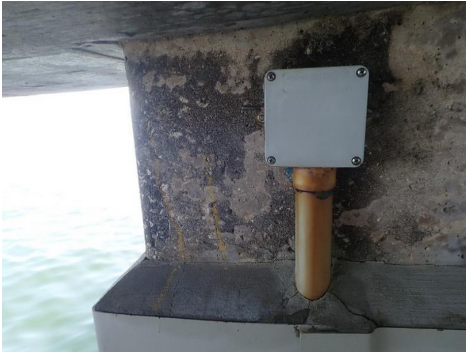
Figure 113. Cracking on pile (Pile 144-4)
