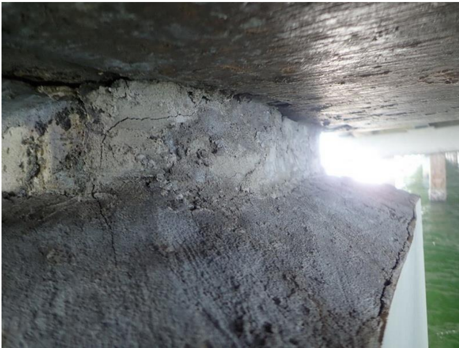
Figure 112. Parge coat cracking, no pile cracking noted (Pile 137-4)
