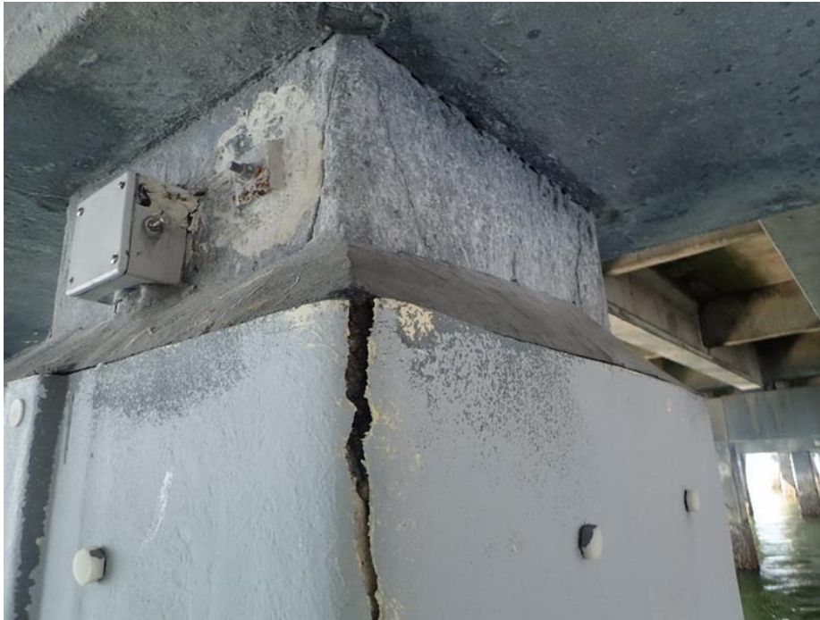
Figure 73. Split pile jacket and multiple vertical cracks on pile (Pile 44-5)
