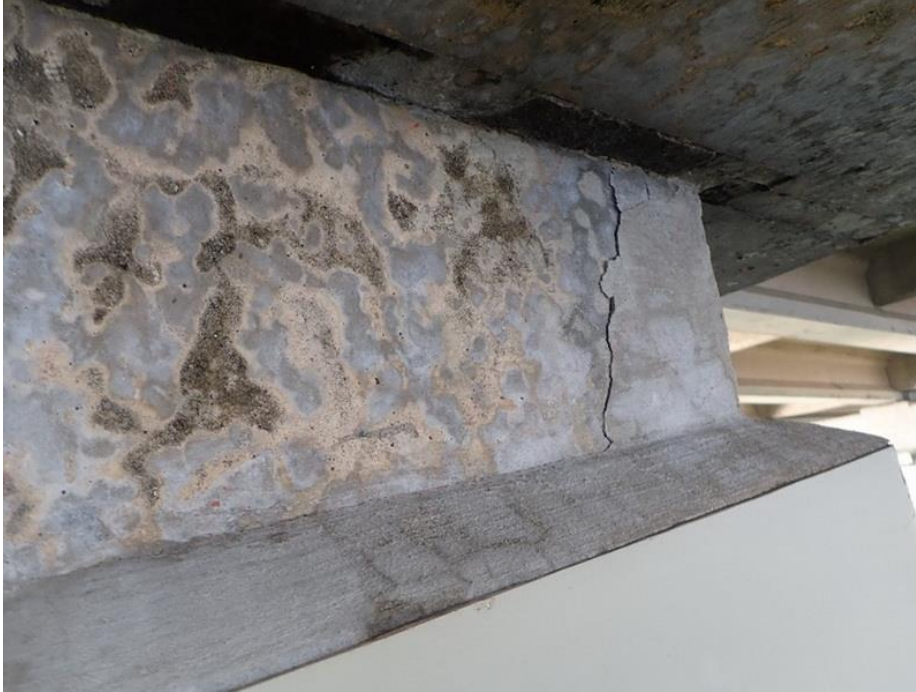
Figure 109. Cracking of pile (Pile 94-3)
