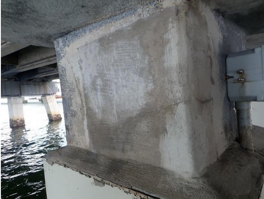
Figure 101. Cracking in repair of pile (Pile 304-4)
