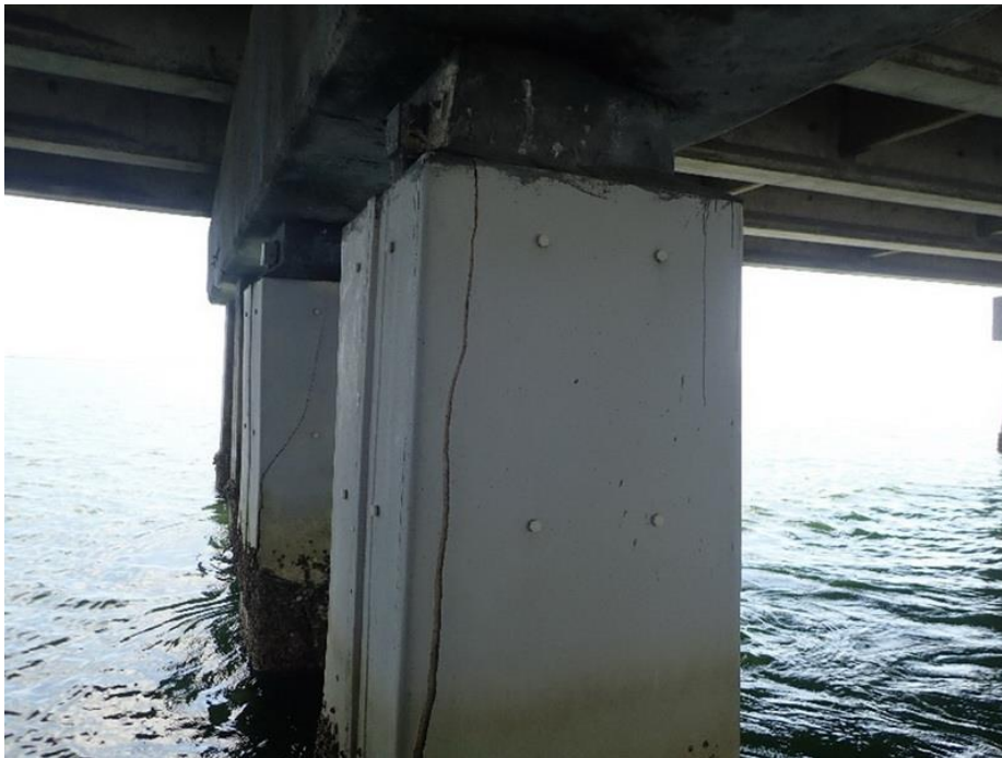
Figure 100. Vertical full length splitting of the jacket (Pile 289-5)
