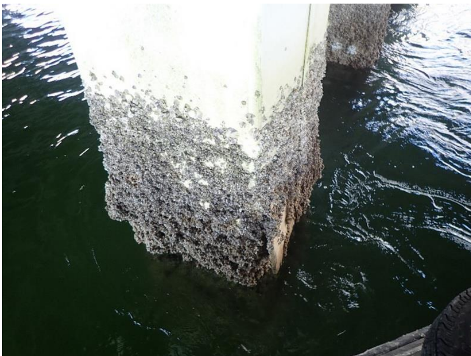
Figure 72. Split pile jacket near waterline (Pile 14-4)
