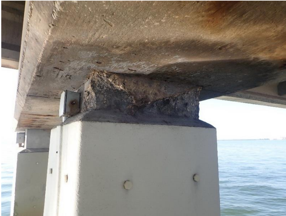
Figure 107. Spalling of pile (Pile 85-4)
