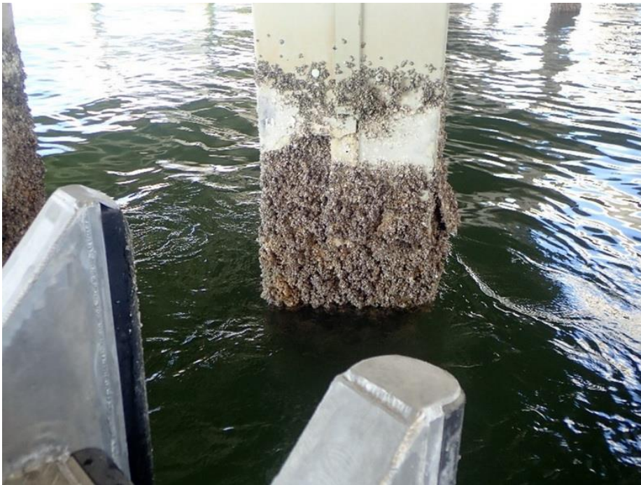
Figure 104. Missing bottom of jacket (Pile 46-3)
