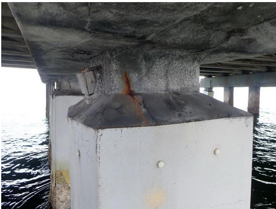
Figure 98. Cracking measured up to approximately 50 mil wide with corrosion staining (Pile 270-2)
