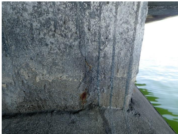
Figure 17. Example of vertical cracking exhibiting minor rust staining (Pile 236-7 shown)
