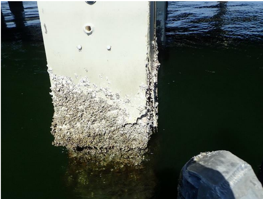
Figure 88. Vertical splitting of jacket (Pile 138-8)
