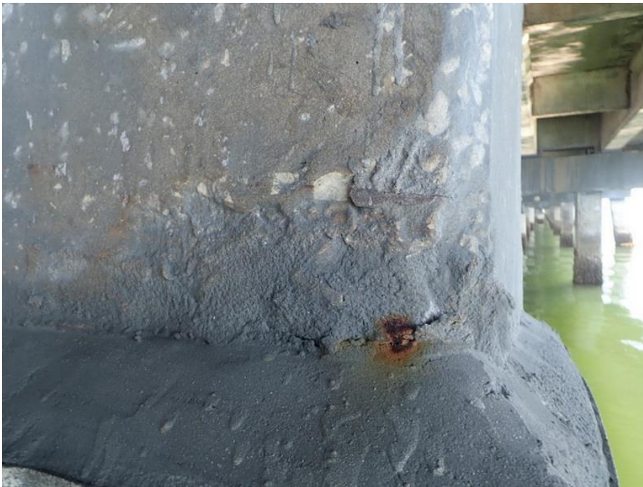
Figure 84. Minor spall on the SW corner top that was metalized over (Pile 123-8)
