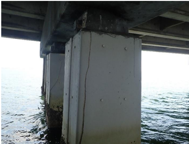
Figure 14. Full-height cracking of fiberglass jacket (Pile 289-5 shown).
