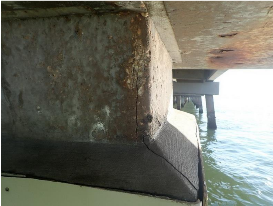
Figure 111. Corner cracking of pile (Pile 106-7)
