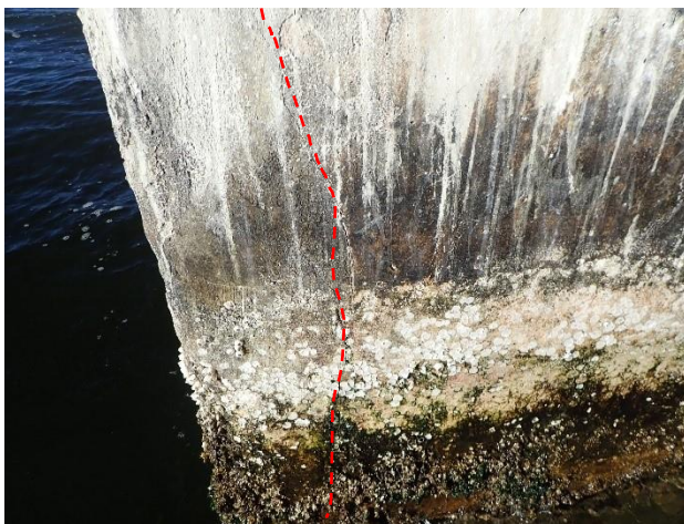
Figure 27. Representative vertical cracking extending upward from the MGL.
