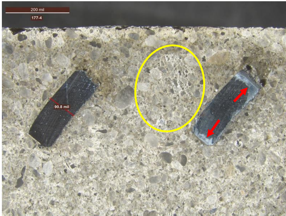
Figure 59. Sample 177-4. Close-up view of zinc mesh shows its condition and thickness measurements. Very localized corrosion and minor section loss were observed. Red arrows indicate locally corroded zinc. White efflorescence was also observed on the lapped section (yellow circle).
