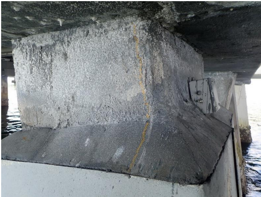
Figure 96. Vertical cracking of the pile (Pile 236-7)
