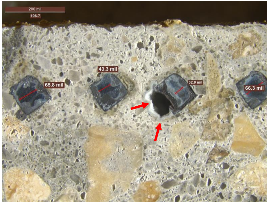
Figure 65. Sample 106-7. Close-up view of zinc mesh shows its condition and thickness measurements. Widespread corrosion and significant section loss were observed. Red arrows indicate white deposits suspected to be zinc corrosion product.
