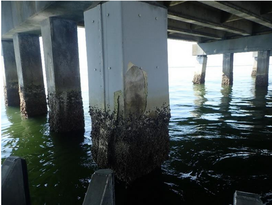
Figure 77. Jacket splitting and missing around lower perimeter of pile (Pile 73-5)
