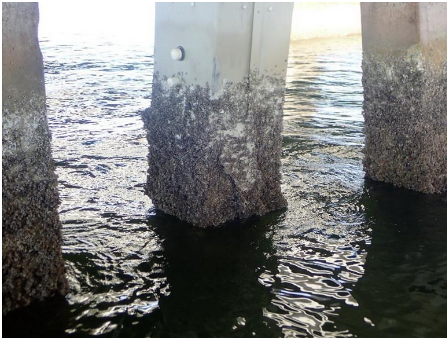
Figure 108. Jacket broken at the bottom Pile 94-3)
