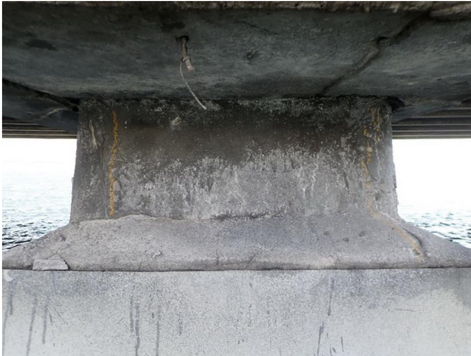
Figure 97. Two vertical cracks of the pile measured up to approximately 5 mil wide (Pile 263-1)
