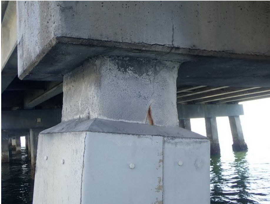
Figure 71. Vertical cracking with rust staining extending upward from top of pile (Pile 12-1)
