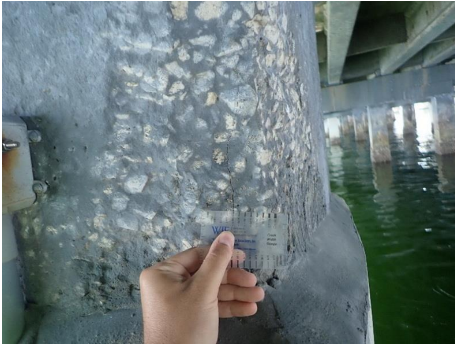
Figure 91. Cracking measured up to approximately 20 mil wide and spalling of pile (Pile 190-6)
