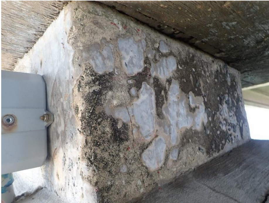
Figure 105. Cracking measured up to approximately 25 mil wide (Pile 82-6)
