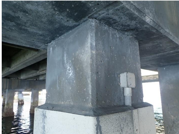
Figure 19. Metalizing overspray observed on pile (Pile 14-4 shown)
