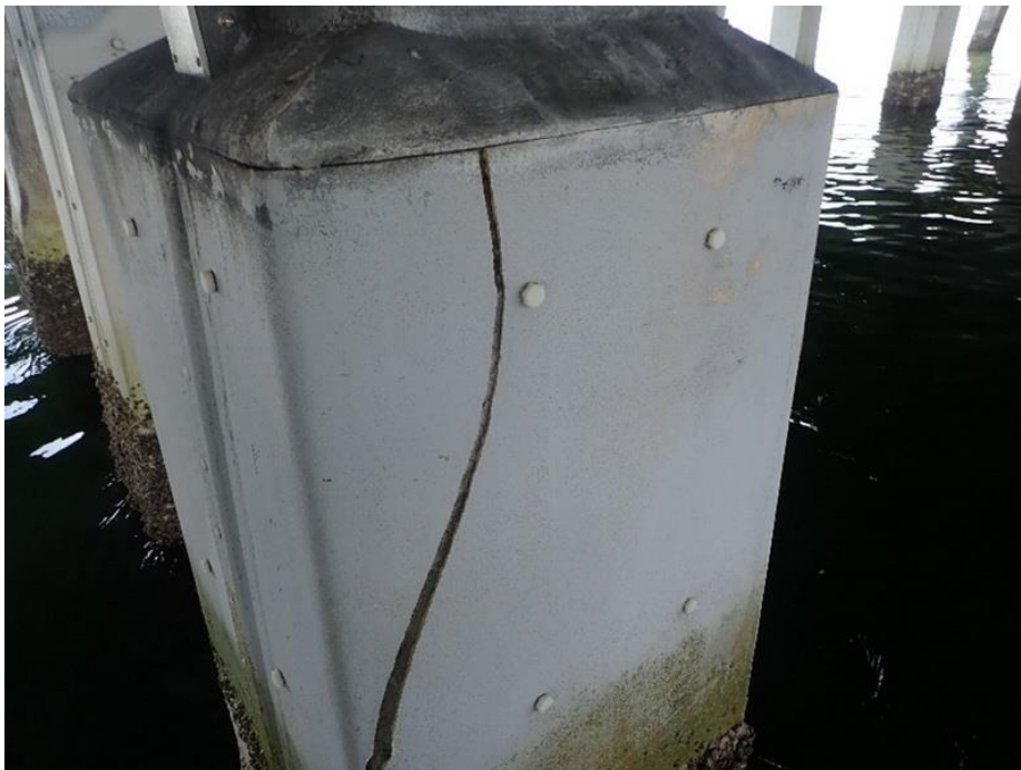
Figure 92. Vertical cracking of jacket (Pile 191-3)
