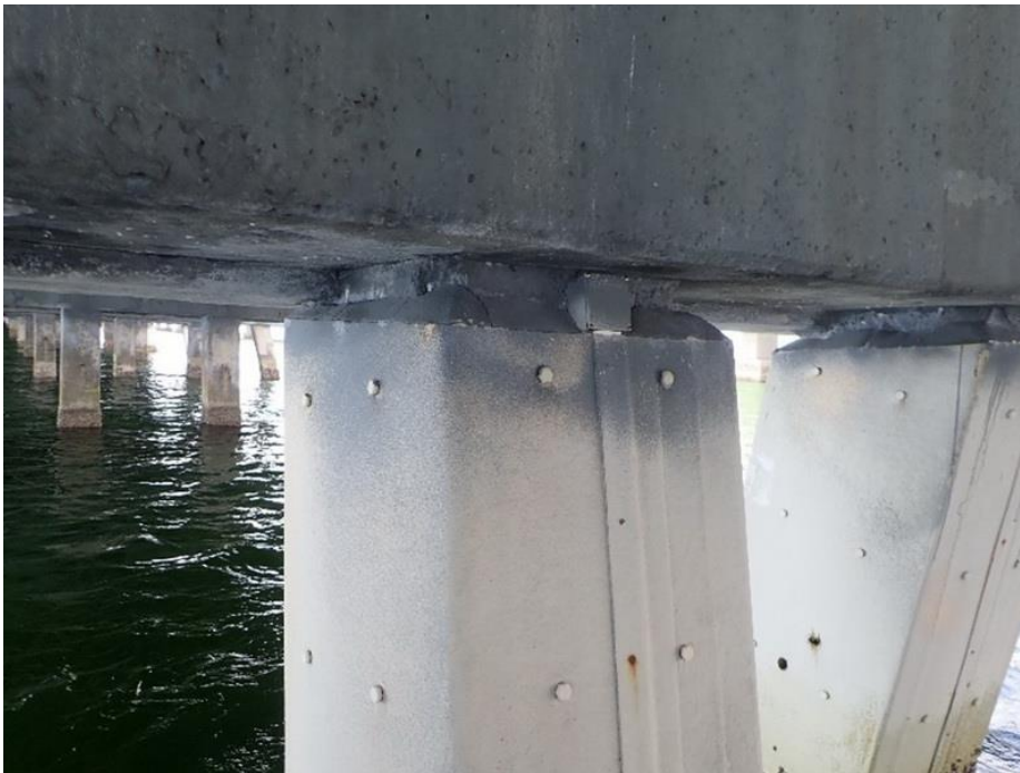
Figure 102. Cracking in repair on top of pile (Pile 308-5)
