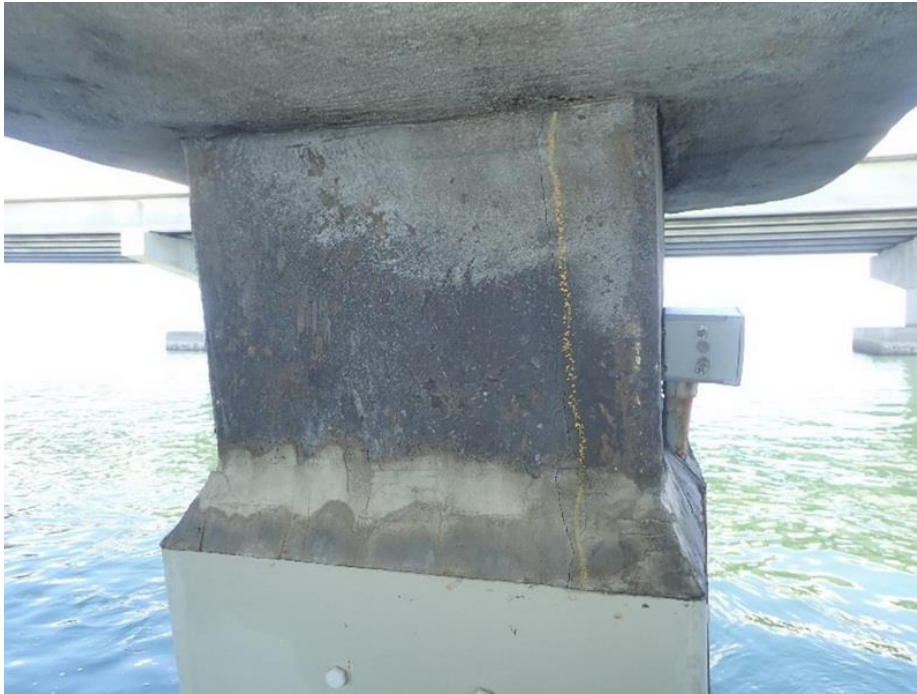
Figure 93. Repair and cracking measured up to approximately 30 mil wide (Pile 198-1)
