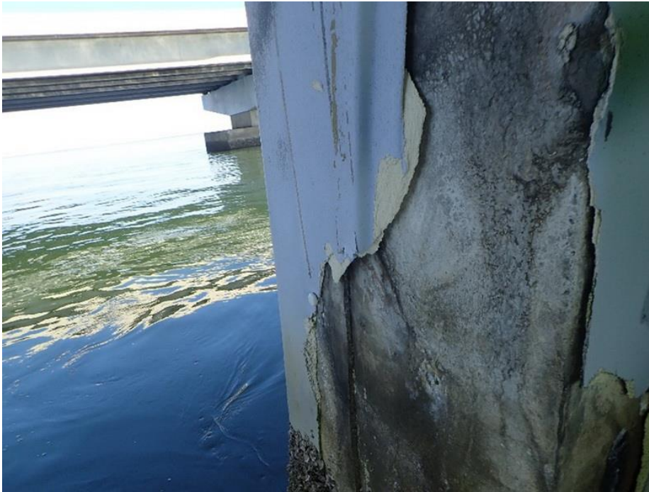
Figure 83. Exposed grout exhibiting staining and cracking (Pile 120-1)
