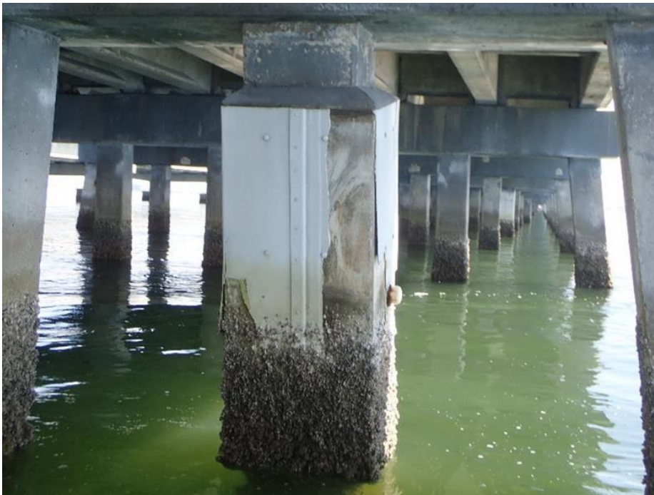
Figure 80. Significant distress of jacket (Pile 105-9)
