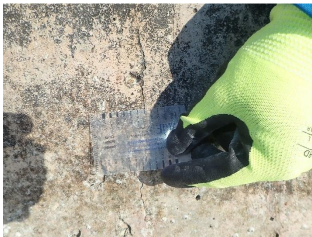
Figure 28. Crack width gauge indicating an approximate crack width of 25 mil.
