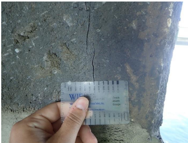
Figure 16. Typical vertical cracking propagating upward from top of pile at corner (Pile 198-1 shown)
