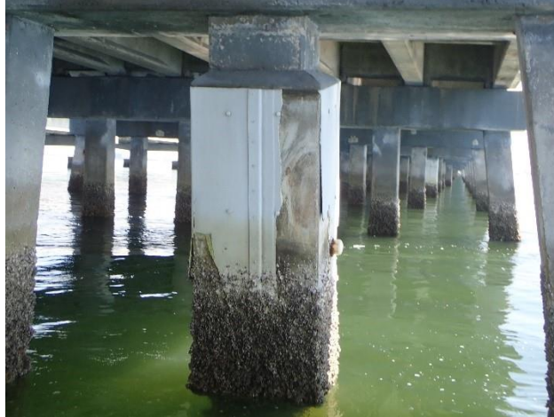
Figure 15. Sections of fiberglass jacket broken off entirely (Pile 105-9 shown)
