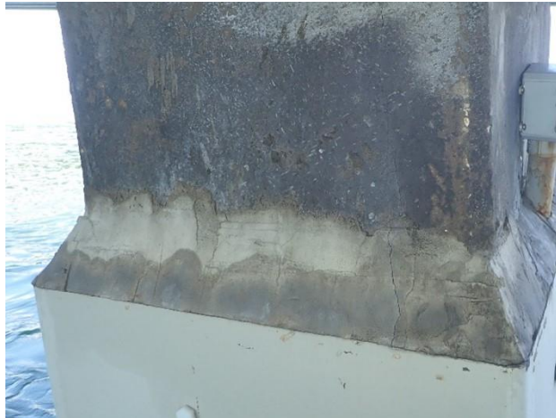
Figure 18. Cracking of sloped grout material above jacket (Pile 198-1 shown).
