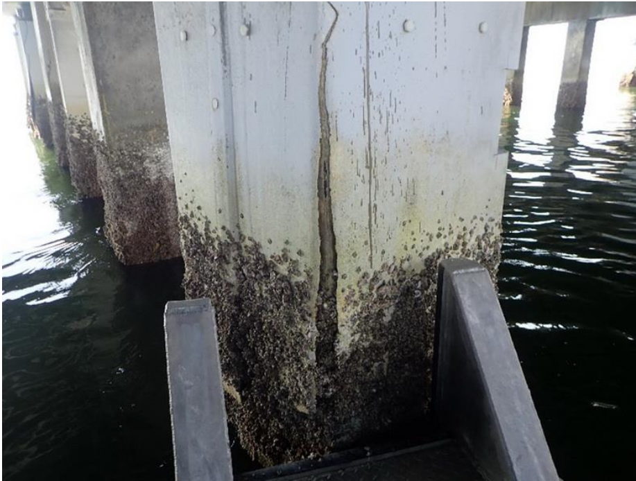
Figure 75. Vertical splitting of jacket (Pile 53-3)
